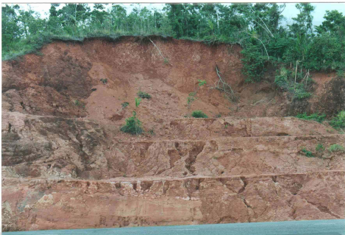
Figure 2.10 Unstable road cutting near Galoa on the Suva-Nadi Highway. Failure is translational, involving residual soil sliding along an irregular, steeply-dipping interface with underlying weathered bedrock, and compounded by shallow rotational movements in the displaced debris mass.
