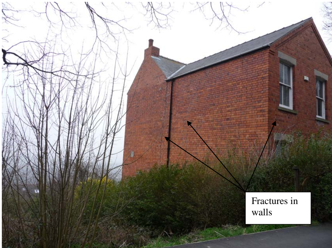
Figure 5. Vertical cracks in brickwork of a house walls indicating ground movement. Carline Road, Lincoln [497147 371869].
