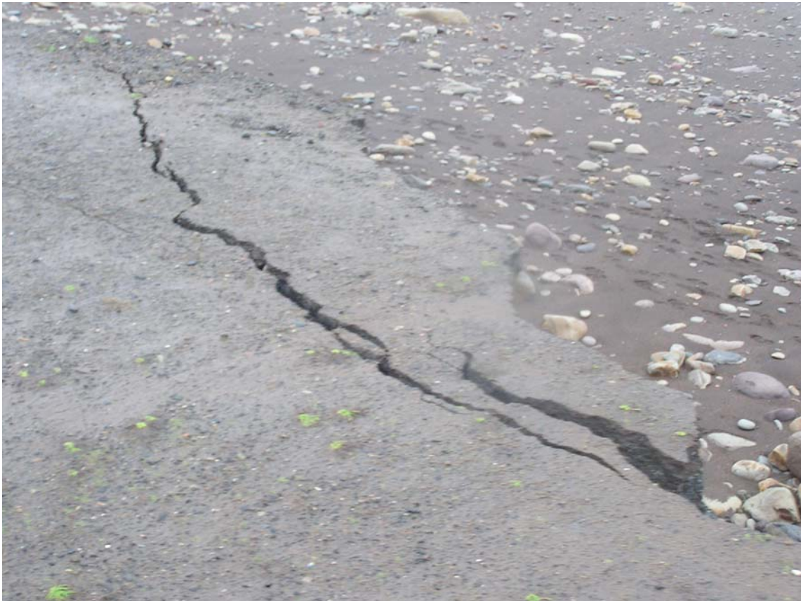
Figure 10. Tension cracks immediately to the north of Landslide C (Photo: BGS, 03/01/07).
