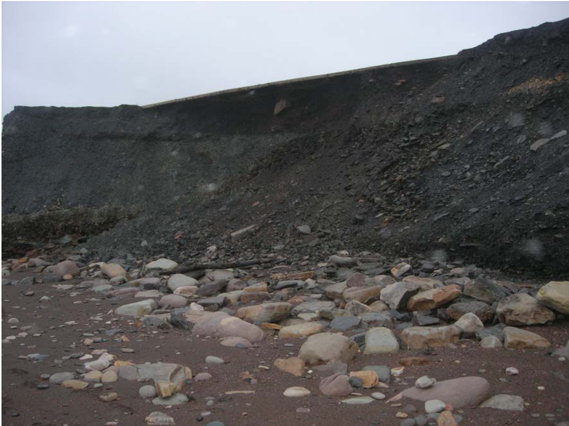
Figure 9. Landslide C undercutting the concrete coastal footpath at NGR 296727 518349. (Photo: BGS, 03/01/07).
