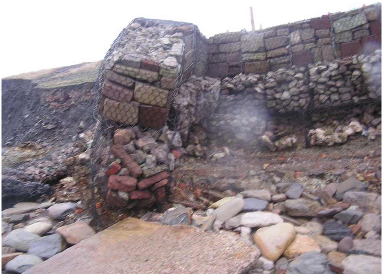
Figure 12. Damage to gabion wall at southern end of beach [NGR 96696 18300] (Photo: BGS, 03/01/07).
