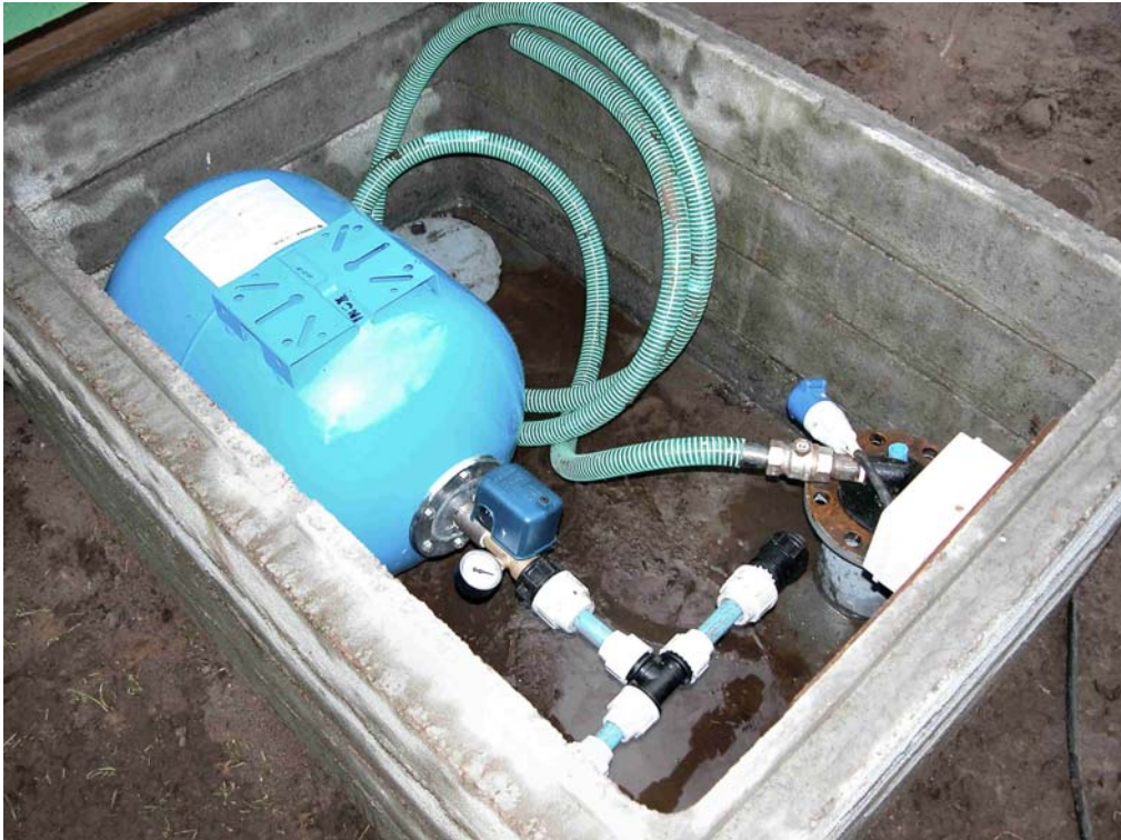
Figure 22 Mark Farm chamber detail, with pressure vessel
