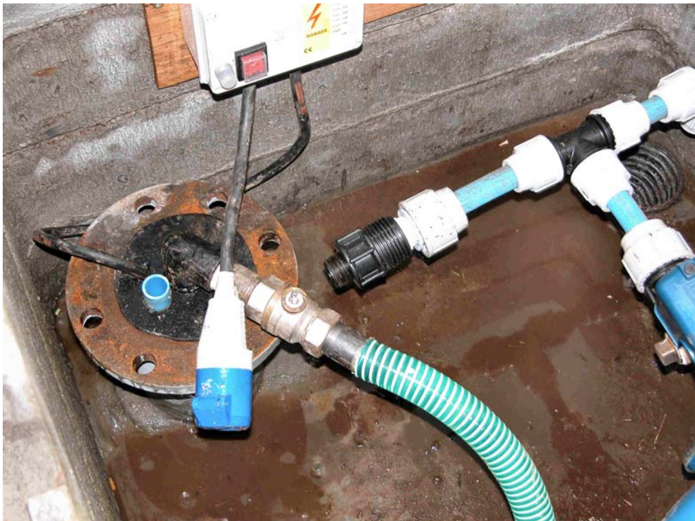
Figure 23 Mark Farm well head
