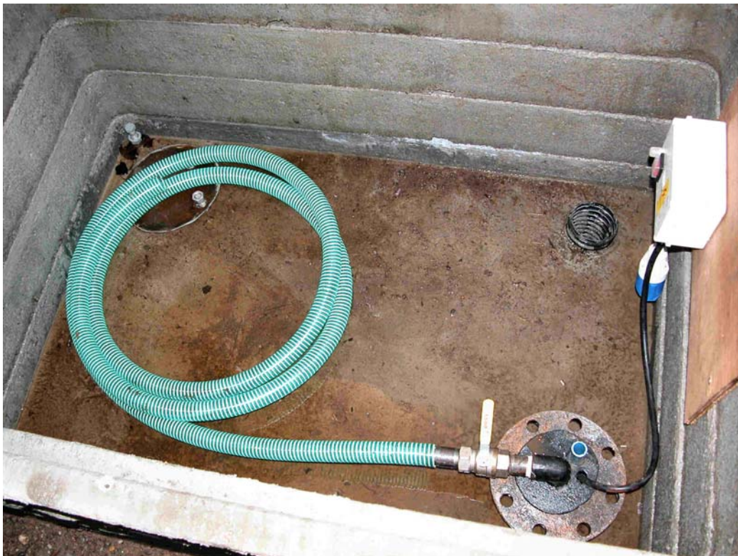
Figure 16 The completed surface chamber with the borehole in the bottom right corner
