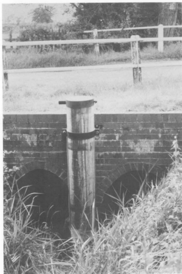
Plate 2.2 Stilling well positioned between twin culverts, Wingrave
