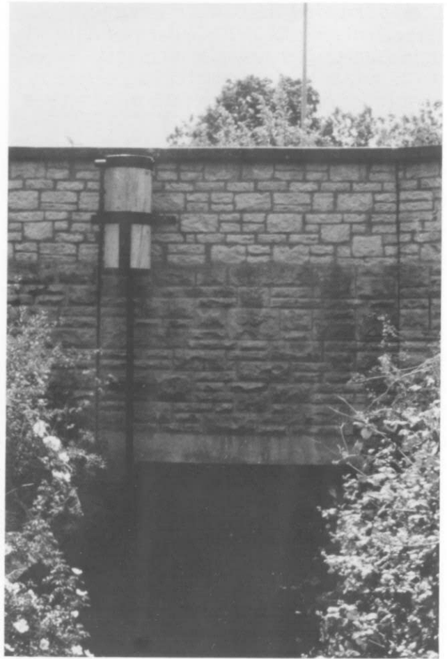
Plate 2.1 Small-diameter pipe used to minimise obstruction to the flow, Bicester
