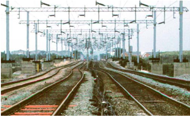
Figure 3. Lateral and vertical movements of the Crewe to Manchester railway line over an area of active salt dissolution and subsidence. Note the pylon bases with vertical adjustment and the lateral movement of the railway line. Photo A.H.Cooper © NERC.
