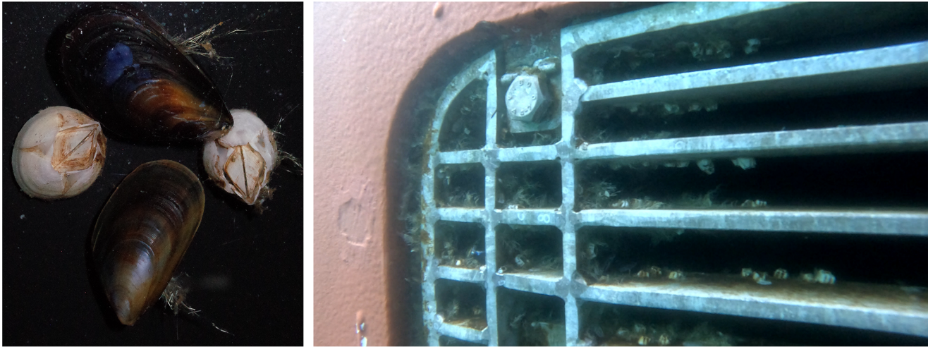
Figure 1. Non-indigenous species assemblage fouling a water intake grill of a research ship located deep into near-shore Antarctic waters in January 2025. Although the anti-foul-treated hull is clean to visual inspection, the water intakes are not similarly (anti-foul) treated, as they supply drinking water. The sizes of the mussels are given in Table I.
