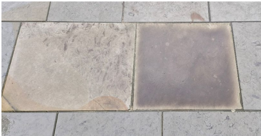
Above: Image showing two typical slabs of the essentially light greyish buff sandstone of unknown identity, when dry. The dark brown discolouration that is extensively developed within the slab seen to the right is more patchily developed in many of the slabs of this type. These slabs in general evidently hold water for a relatively prolonged period of time once wet (cf. the Whitworth Sandstone ).
