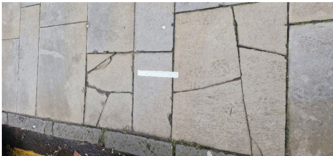
Above: Image showing a damaged section of the sandstone paving at Locality 5 (seen dry); 30 cm ruler for scale.
