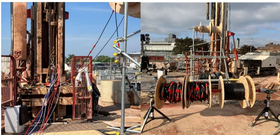
Figure 17 Images of the installation being run into TH0418 showing the MLS lines, the ERT and FO cables
