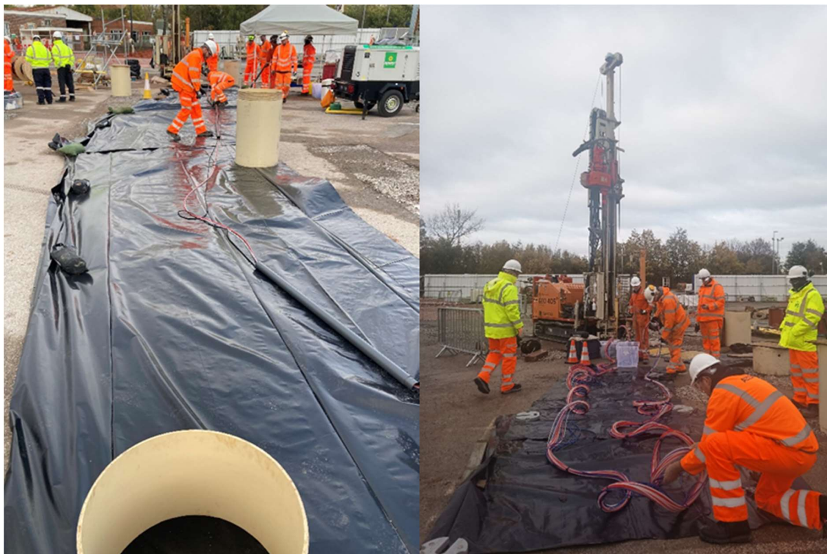
Figure 28 left hand image showing preparation works for running, right hand image shows the end of the install, and all MLS ports run.
