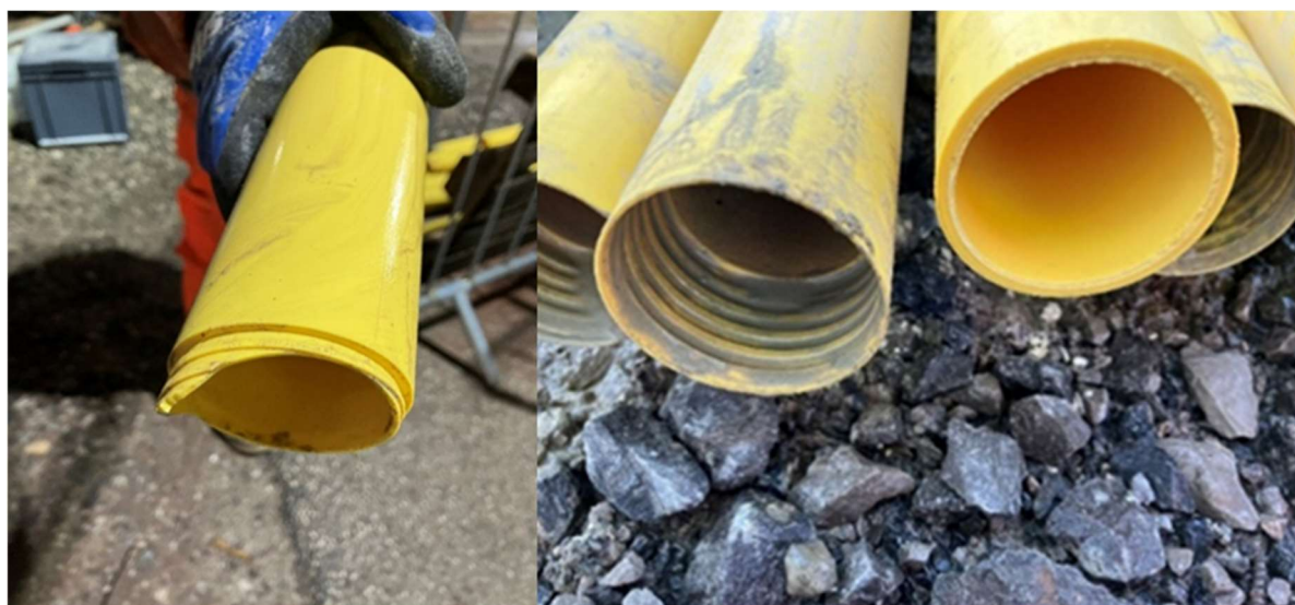
Figure 105 left hand image is of a snapped pin connection of 60 mm tremie pipe, right hand image shows the pin end shearing off completely as a clean break
