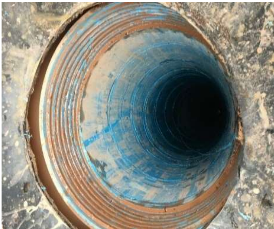
Figure 74 Scoring on the intermediate casing from dropped spanner
