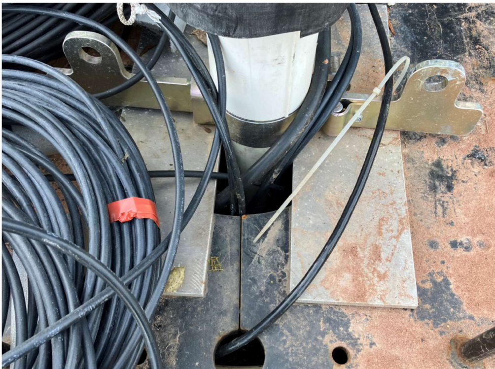
Figure 85 Speed clamp and C plate supporting rising main TH0412
