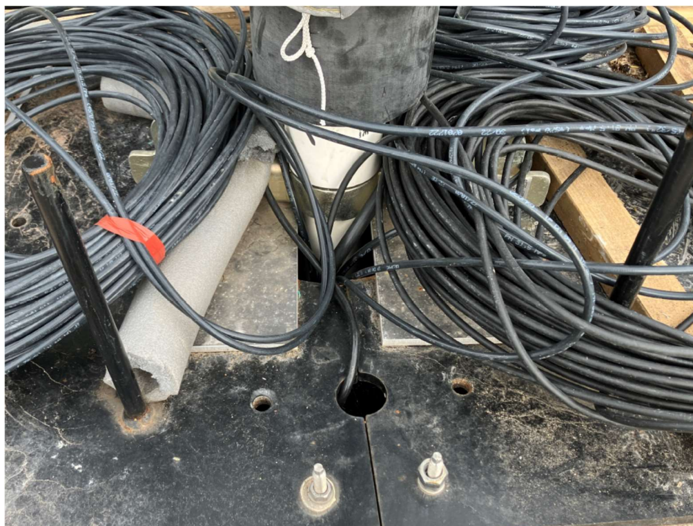
Figure 79 Speed clamp and C plate supporting rising main TH0408
