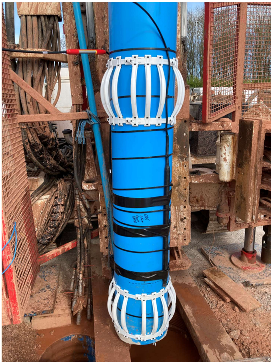
Figure 86 Intermediate 330 mm OD casing being RIH with ERT and FO cables secured to the outside
