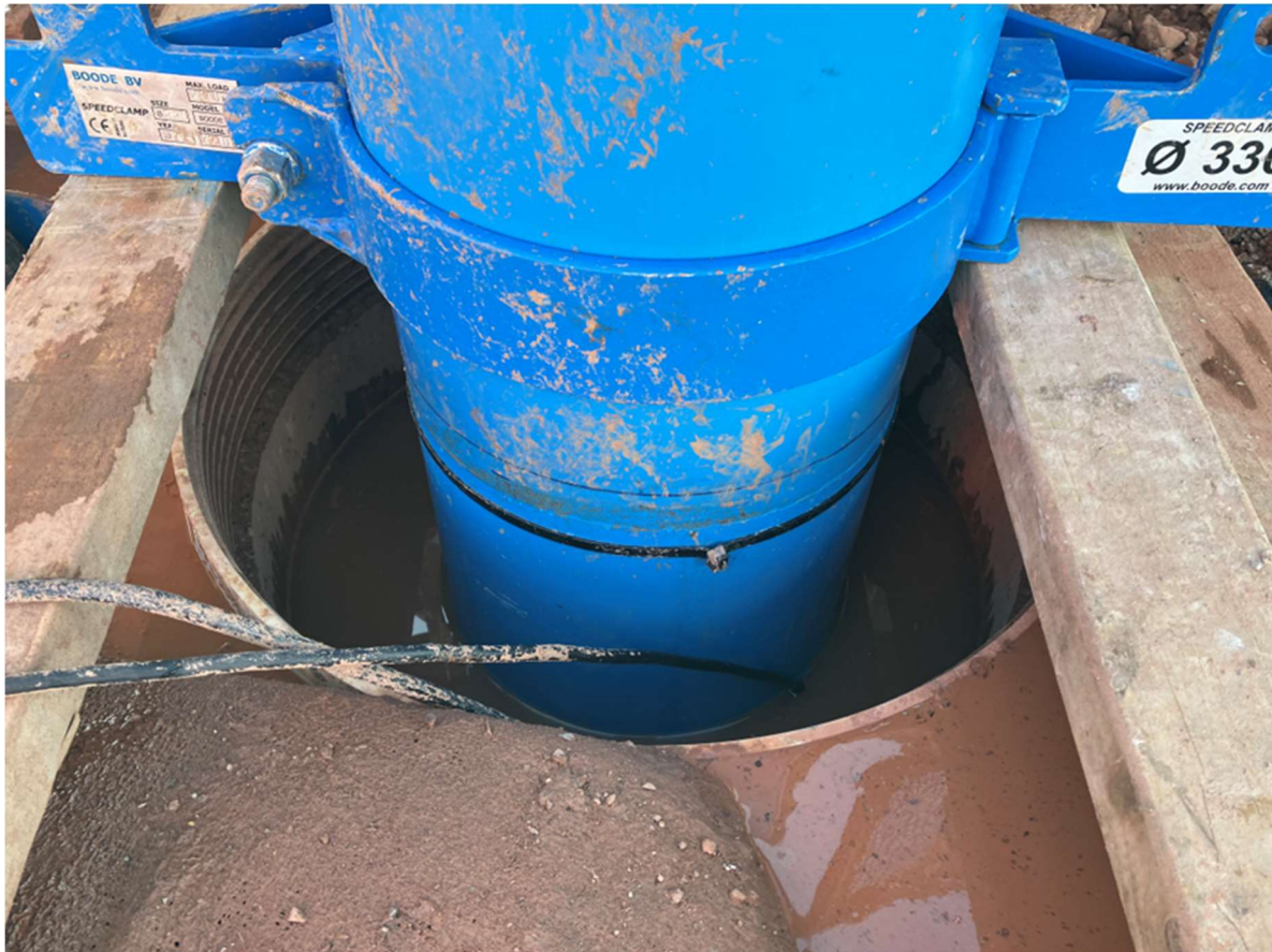
Figure 73 Intermediate 330 mm OD casing installed with ERT and FO, grout level below GL
