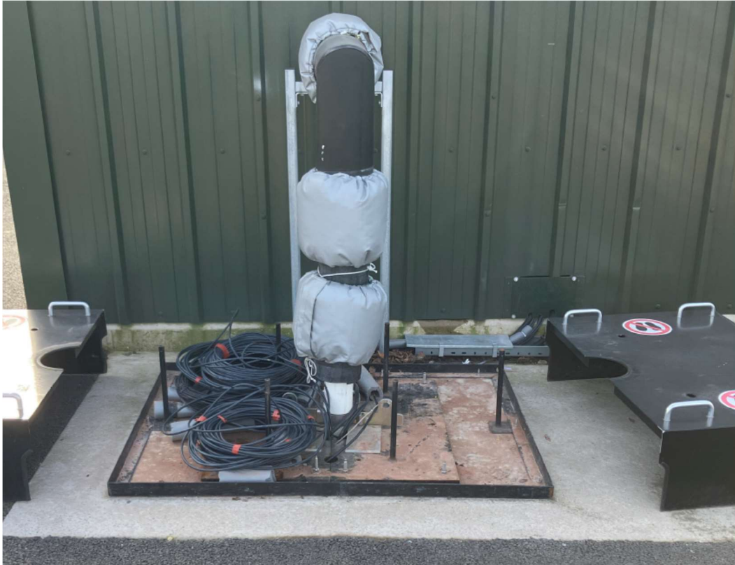
Figure 84 Wellhead status TH0412
