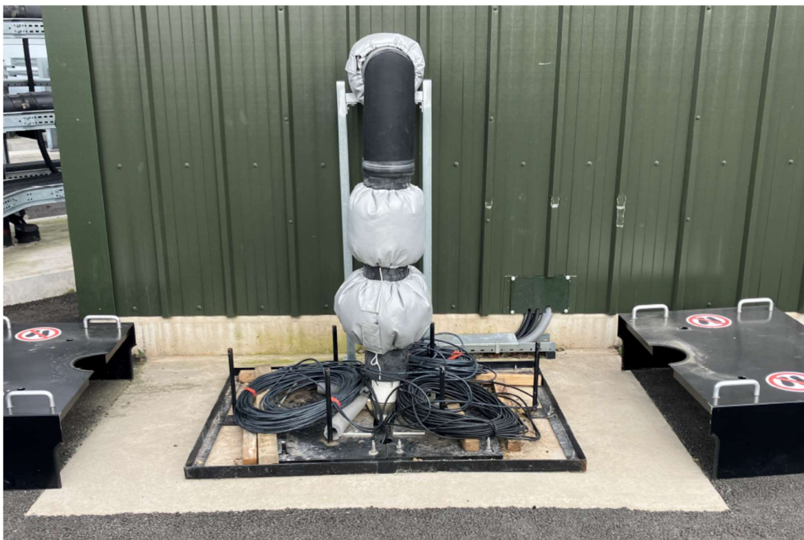
Figure 78 Wellhead status TH0408
