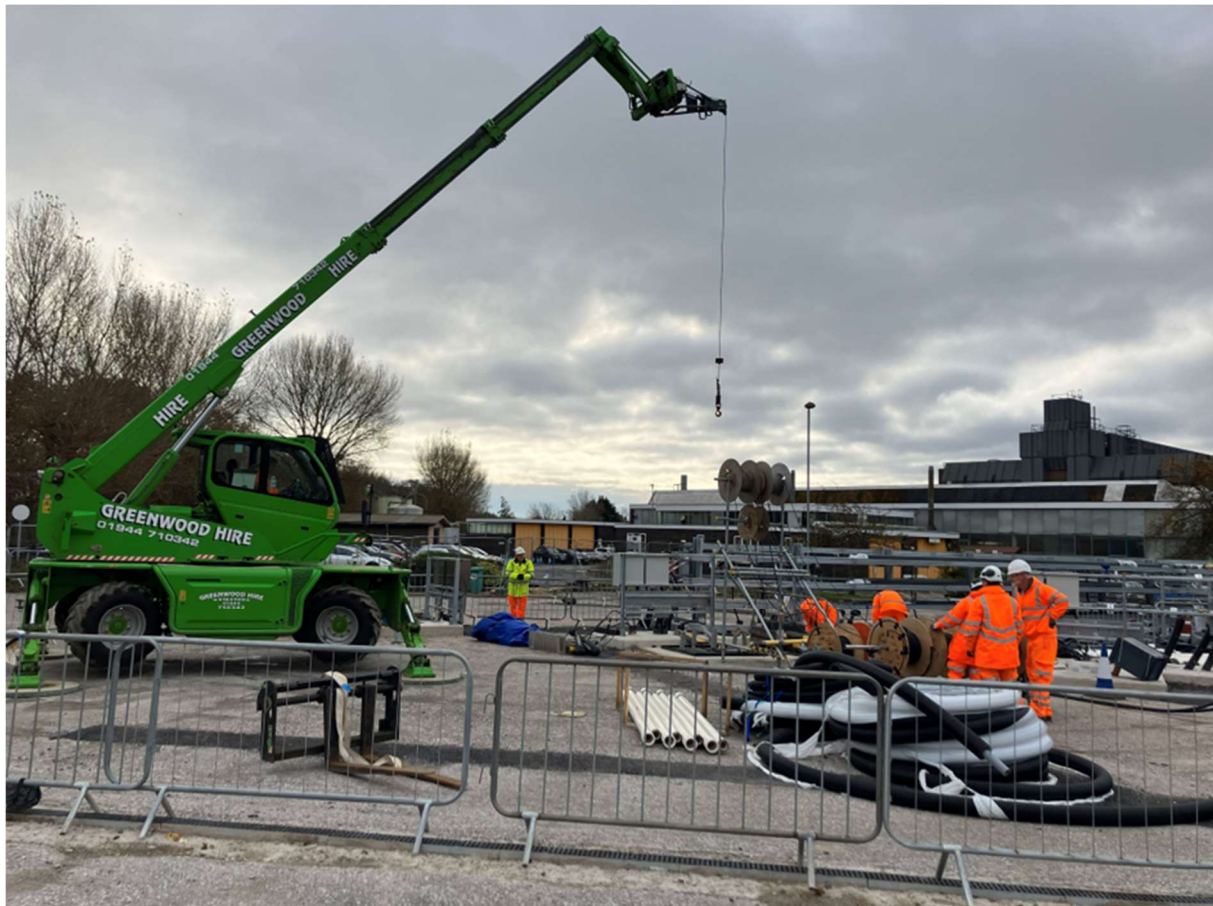
Figure 82 Setting up in readiness for running the packer and pump assembly into TH0412
