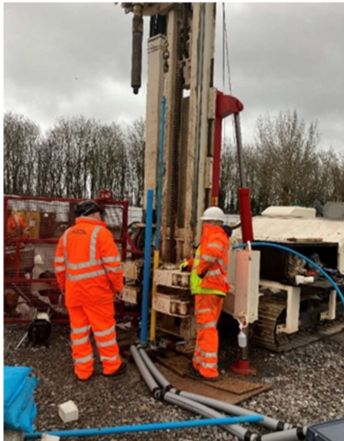
Figure 111 75 mm installation pipe run. 30 mm tremie (blue) being run through the 60 mm tremie (yellow) to push through a Bentonite blockage during back filling operations.
