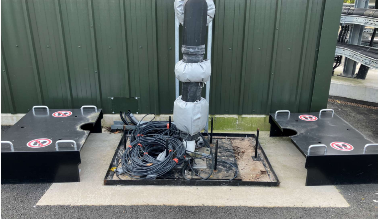
Figure 71 Wellhead status TH0406
