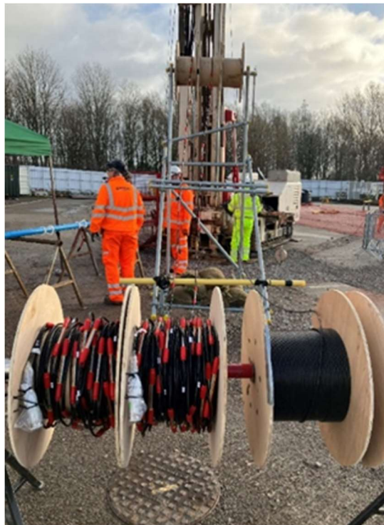
Figure 104 TH0411 installation setup
