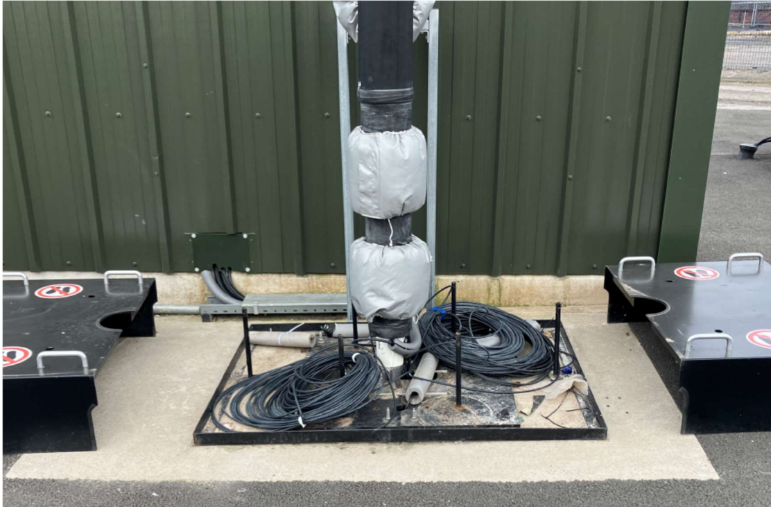
Figure 89 Wellhead status TH0414
