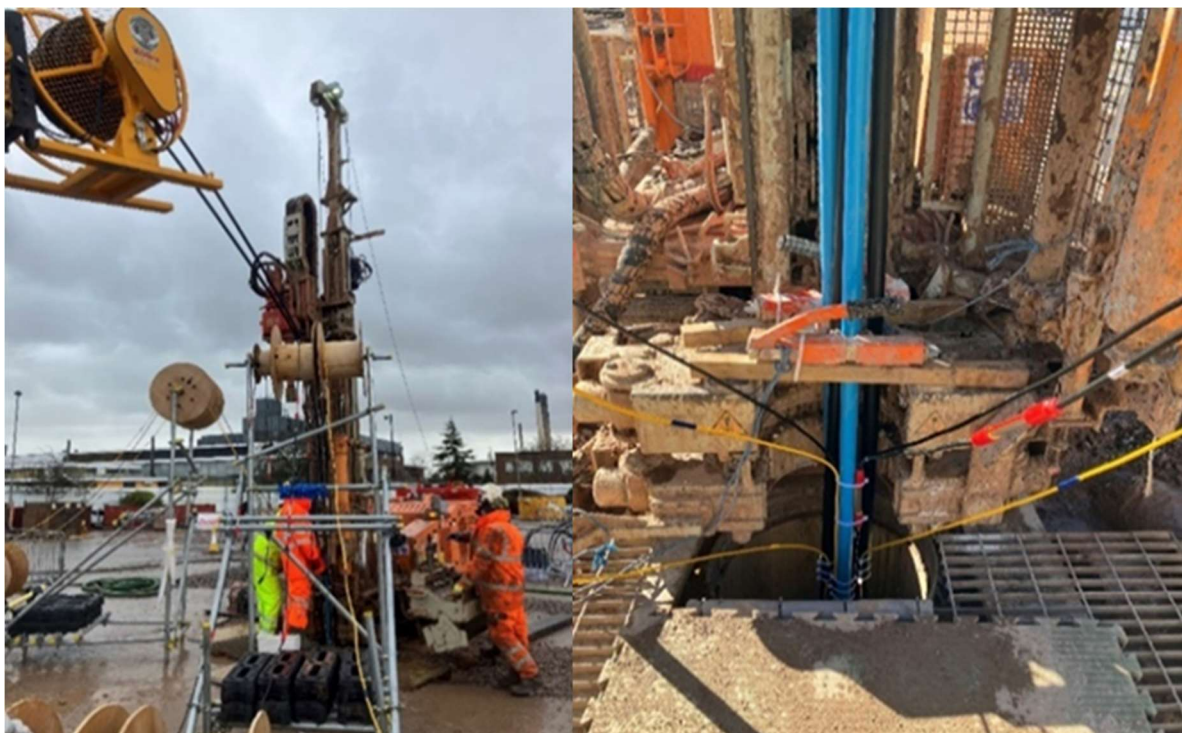
Figure 60 Installation images of the heat exchanger loop, primary and backup tremie pipes and all the cables / cable management as its RIH
