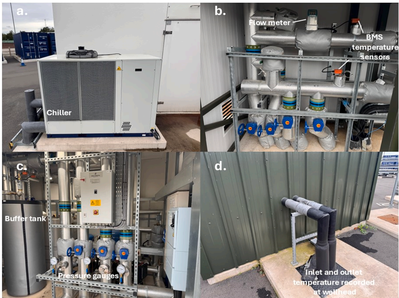
Fig. 3. Pictures of the equipment used during testing: (a) chiller for the heat extraction mode borehole heat exchangers, (b) control valves between the surface piping and borehole heat exchangers, (c) control valves between the chiller/heater and outer pipework, and (d) connection to the wellhead for the inlet and outlet fluid.
