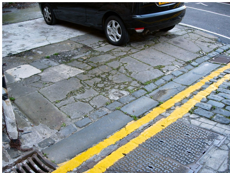
Photo 18. Damaged area of sandstone paving with whinstone kerb and gutters in Hill Street North Lane.
