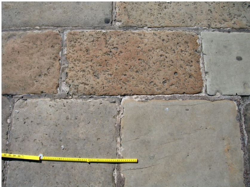
Photo 48. Sandstone paving on the north side of Charlotte Square, showing typical variable appearance ranging from dominantly greyish to reddish-brown colour with variable surface texture from smooth to rippled surface. These variations are typical of the original sandstone paving found throughout in the Edinburgh New Town. The pale grey slab (centre right-hand side) is a later replacement sandstone (note the straight sawn edges). Scale ruler is c.750 mm long.
