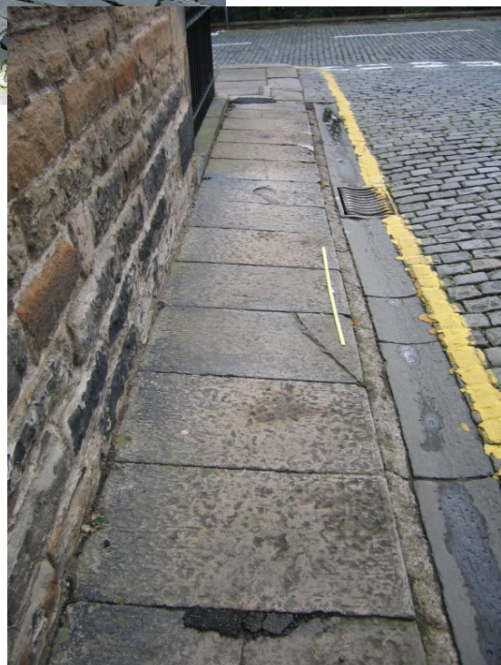
Photo 25. Typical sandstone paving with a single row of large slabs aligned perpendicular to the kerb. The flagstones have a naturally rough surface due to the presence of ripple bedding laminae. The original kerb has been removed and replaced by concrete, and a dished whinstone gutter and setted roadway are present. (Carlton Terrace Lane).
