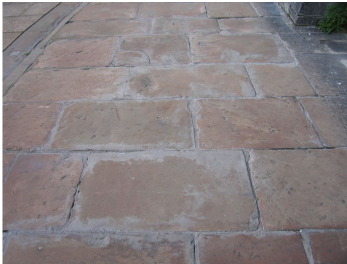
Photo 29. Part of the sandstone pavement on Regent Road recently re-laid following utility maintenance works. The slabs have been crudely replaced using a grey cement mortar, and some have been damaged.
