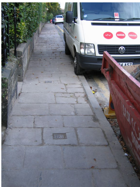
Photo 4. Illustration of the modern pressures on traditional paving. The parking of vehicles on the pavement edge causes flagstones to break. (Ann Street).
