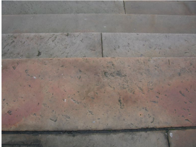
Photo 36. Detail of main entrance steps, General Register House, showing reddish-brown patina to worn surfaces, with pitted surface caused by effect of ripple bedding. These features are very similar to much of the remaining original sandstone paving present throughout the Edinburgh New Town, and is typical of local 'Hailes-type' sandstone.
