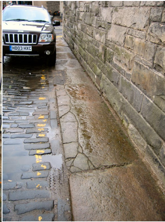
Photo 12. Typical damage to natural sandstone paving caused by parked vehicles mounting the footway. (Lynedoch Place Lane).
