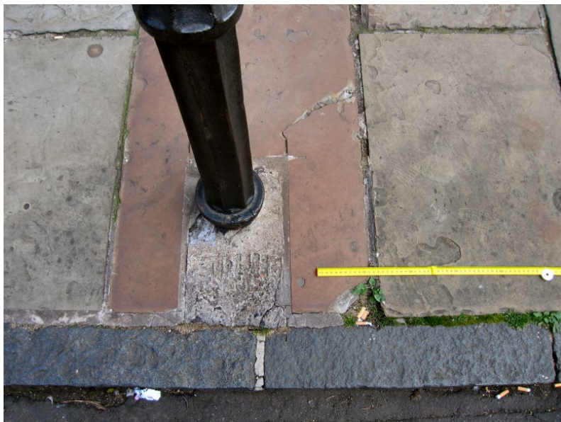
Photo 52. 'Recent' installation of bollard into sandstone paving, St Stephen Place, with over-large sawn area patched using cement and cracks to the sandstone slab.
