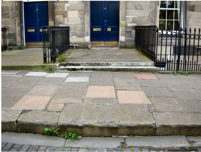
Photo 23. Original sandstone kerb and mounting block, Carlton Terrace. The paving slabs have been replaced by concrete slab. Mounting blocks are present adjacent to a number of the property entrances.
