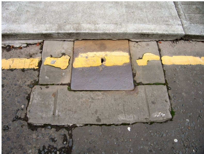
Photo 13. Example of one of the few remaining sandstone surrounds to cellar entrances on Atholl Crescent, on the road adjacent to the pavement. The entrance itself is infilled by a metal plate.
