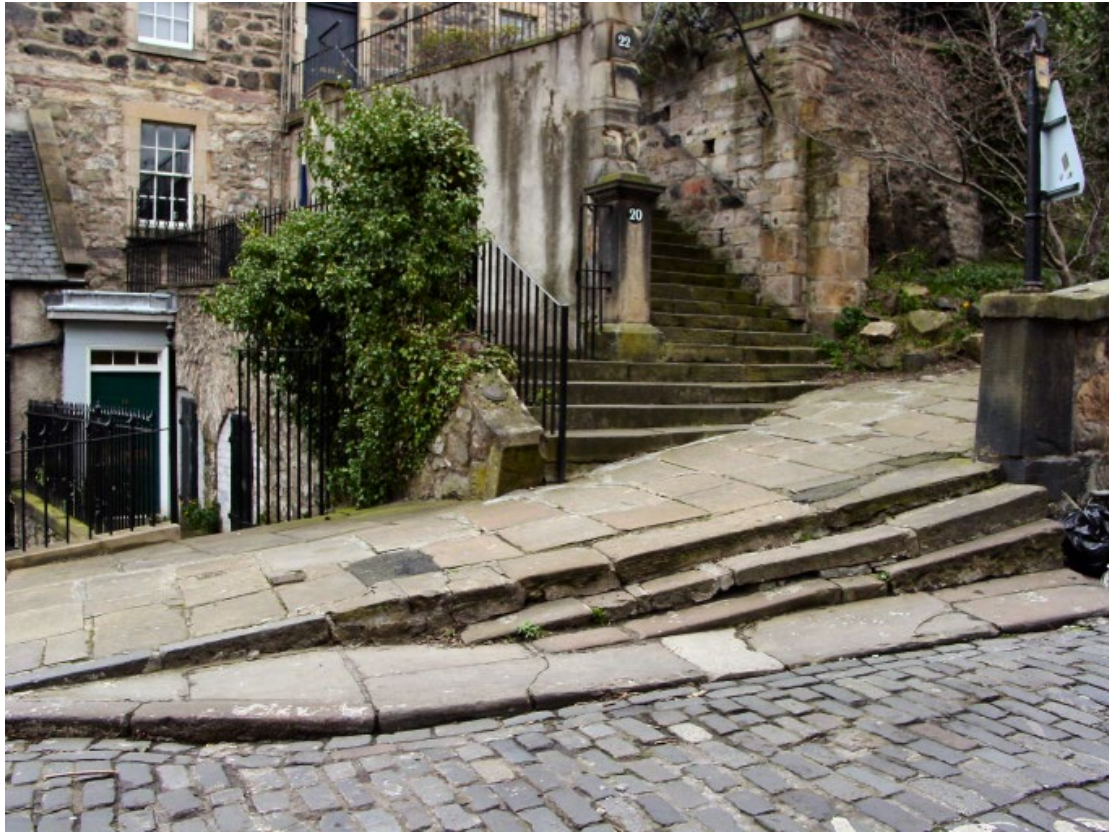
Photo 33. Original sandstone pavement and steps on the north side of Calton Place, with whinstone kerbs and setted roadway. Although the paving slabs are now in poor condition, the continuity of stone materials from roadway, footpath, entrance steps and buildings adds to the character of the historic built environment.
