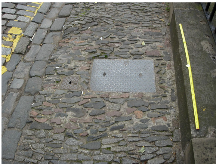
Photo 58. Poor attempt to mimic horonizing following installation of service duct, using a mixture of original material and red whinstone fragments, loosely packed in a cement matrix. South-eastern side of Ainslie Place.
