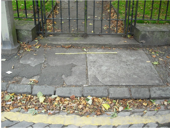
Photo 56. Northern garden entrance, Ainslie Place, with two large sandstone slabs partly covered in asphalt.
