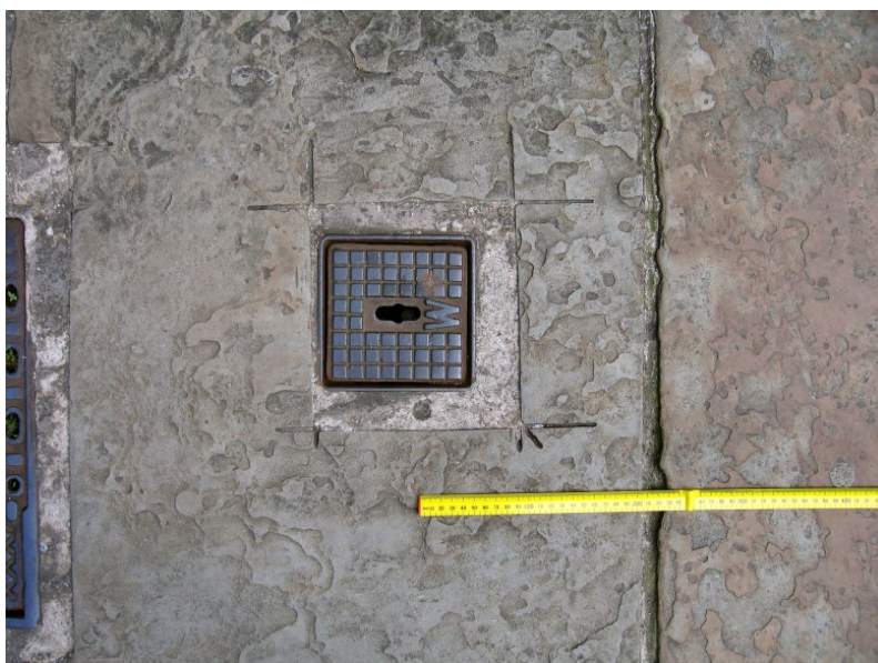
Photo 53. Detail of sandstone paving, St Stephen Street showing installation of utility service point, showing unsightly sawing of slab and cement patching.
