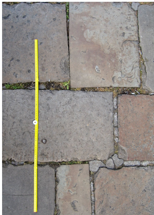
Photo 10. Poor quality re-laid pavement using original sandstone slabs cut with a mechanical saw. Slab edges and joint widths are irregular and the hard cement mortar is broken. Scale is 1 metre (Bells Brae).
