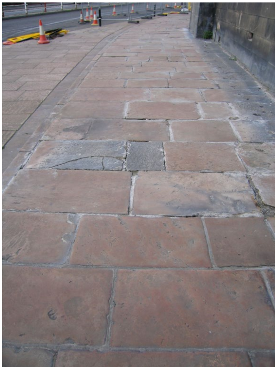
Photo 30. Part of the sandstone pavement on Regent Road recently re-laid following utility maintenance works. The slabs have been crudely replaced using a grey cement mortar, several have been damaged, and the two (now broken) darker slabs in the centre of the image were originally located against the wall on the inside of the pavement, having been re-laid in the wrong position.
