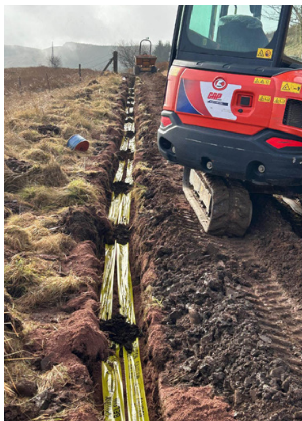
Figure 32 Replacements to the local area networks at Eskdalemuir. BGS © UKRI.
