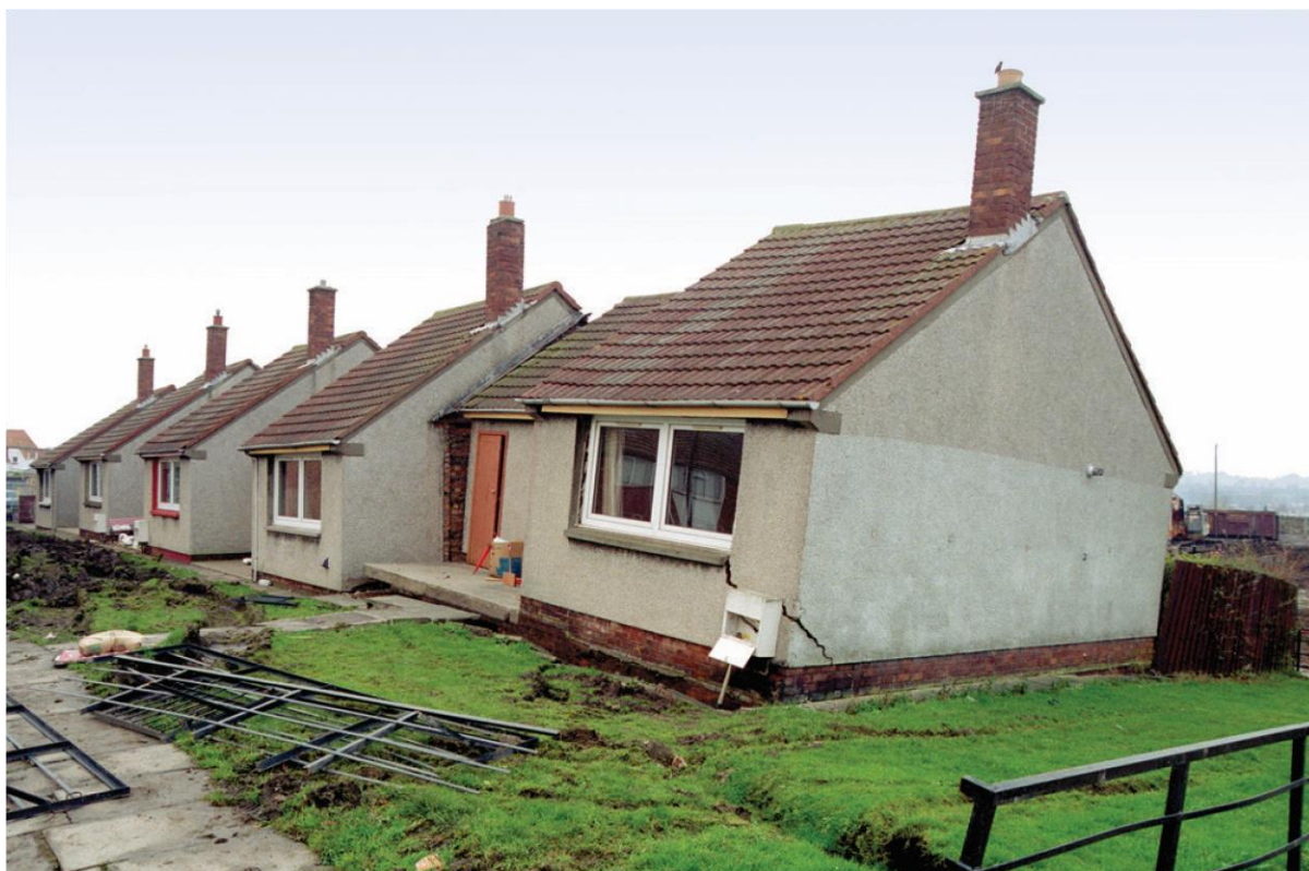
Plate 17 Mining subsidence event early November 2000 to March 2001 at Ferniehill [NT 2940 6920], Gilmerton over the Hurllet (Gilmerton) Limestone mineworkings. Note tilting of cottage on its raft foundation and structural damage to properties, infrastructure and also open cracks in ground (P100365) BGS © UKRI
