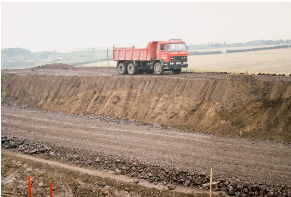
Plate 15 City of Edinburgh Bypass [NT 2685 9090], view south of temporary section during construction showing the Roslin Till, with thrust to right of lorry at sharp basal contact on underlying sands; (P265553) BGS © UKRI
