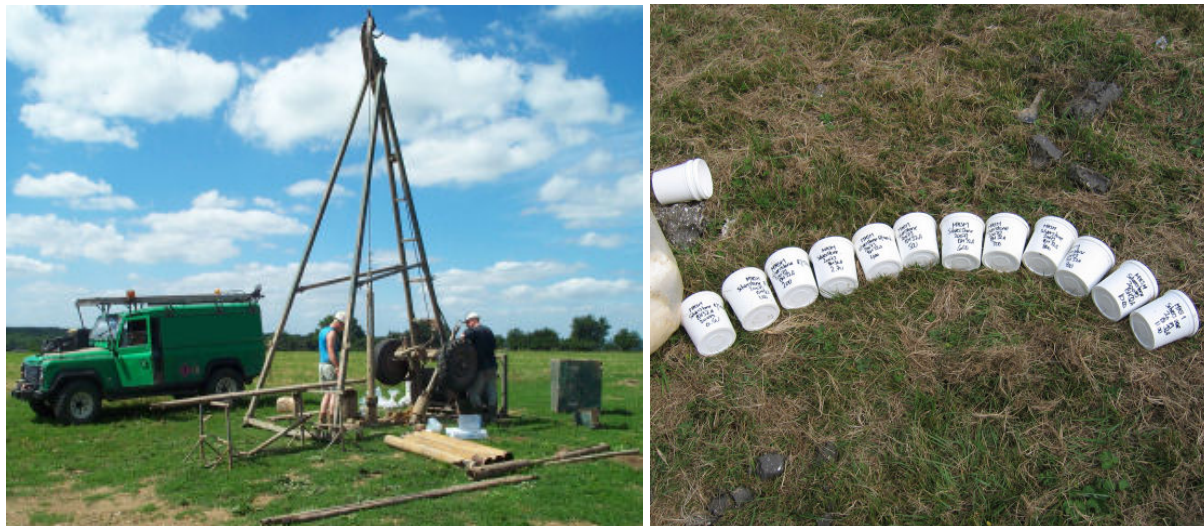
Plate 1 The shell and auger percussion drilling rig, drilling one of the Project boreholes
