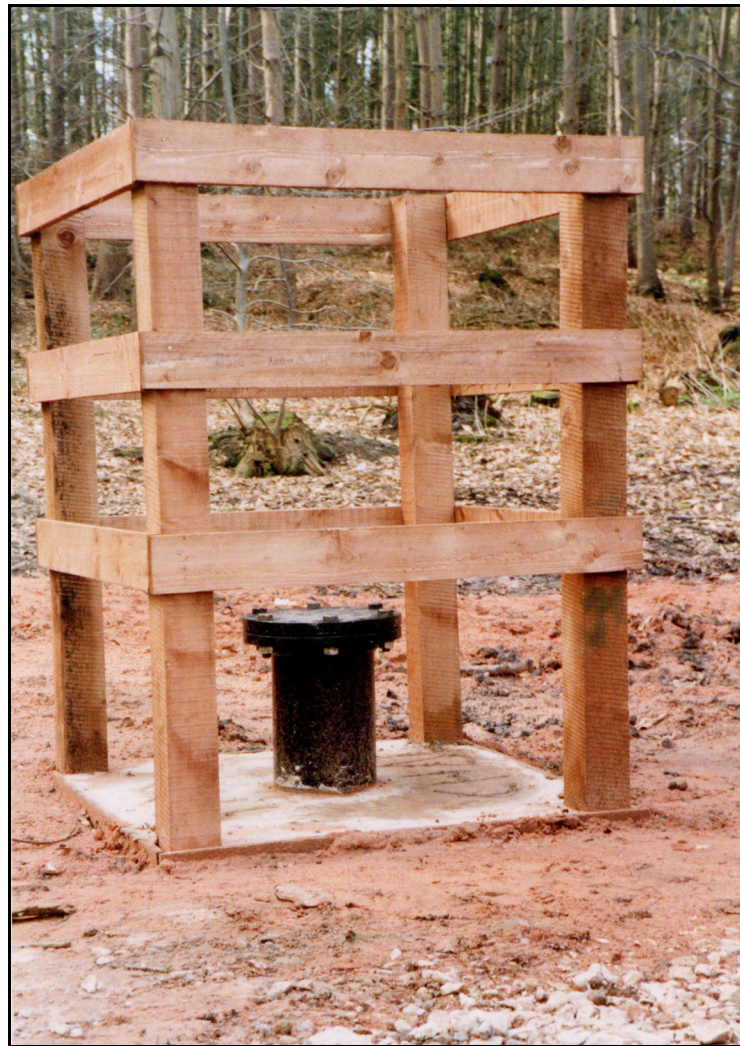
Figure 4.4 Photographs showing the Abbey Arms Wood borehole during construction, including core processing and the borehole after completion (photographs by John Ingram, EA).
