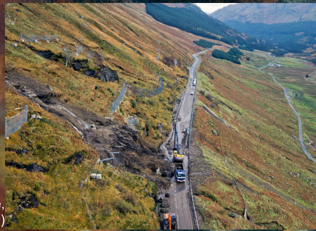
Landslide on the Rest and be Thankful passage, Argyll & Bute, Scotland (Credit: Traffic Scotland)
