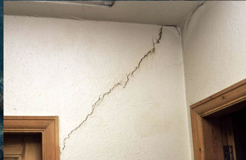
Image: a cracked wall in a subsiding house. Cracks can appear inside, outside, or both, causing extensive property damage. Image credit: BGS
