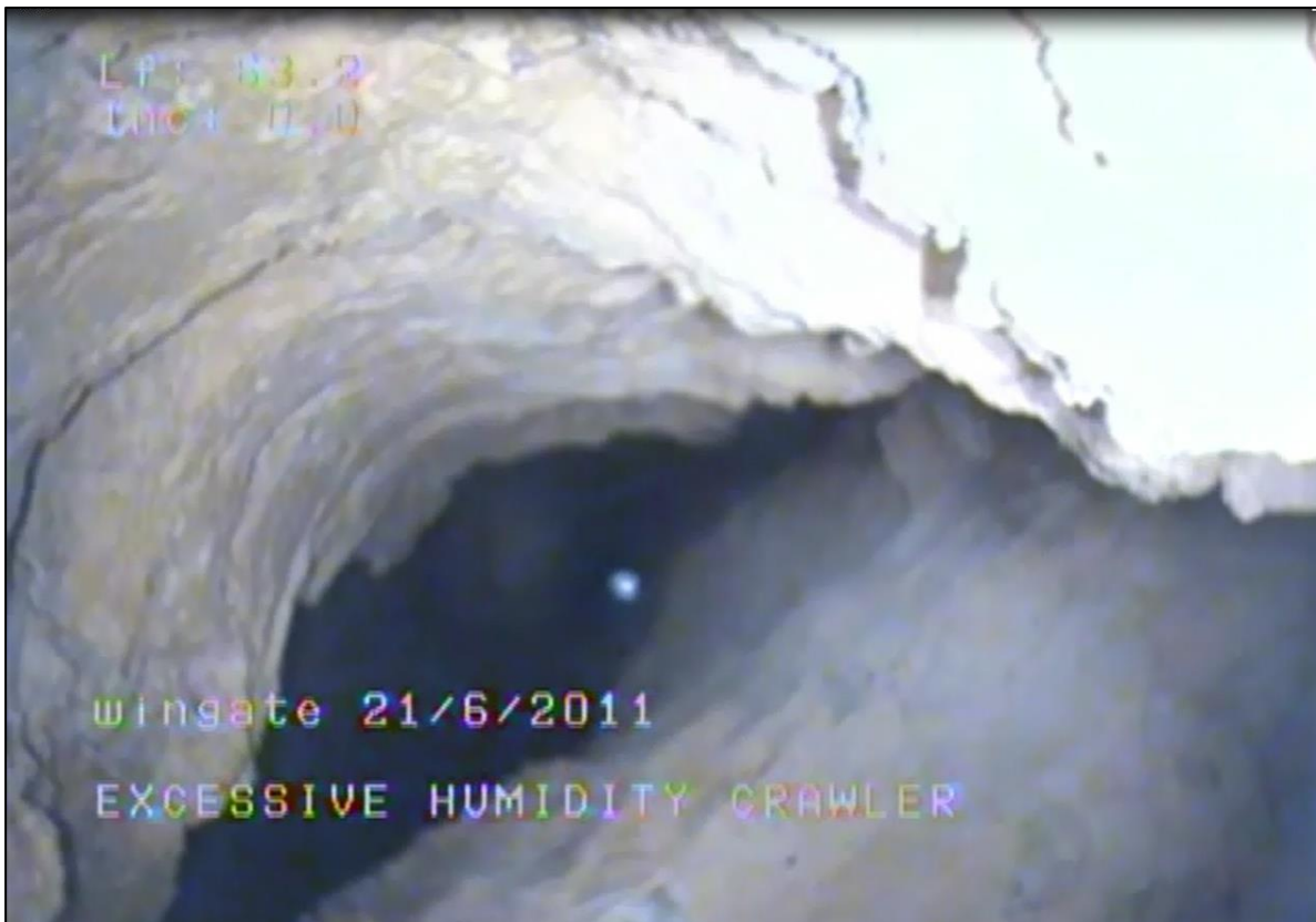
Figure 15. Borehole images of a conduit intercepted by a borehole at Murton Hall Farm Pictures Courtesy of Anglian Water Services
