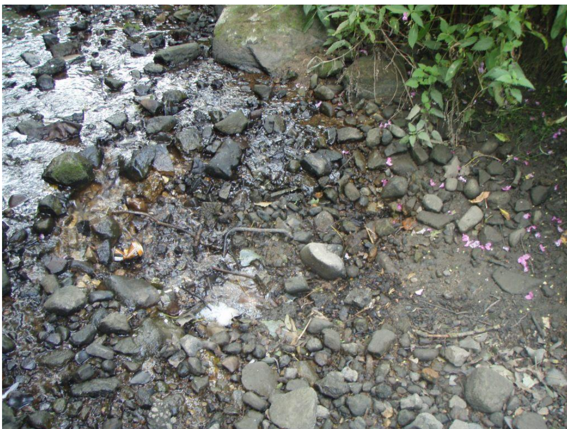
Figure 18. Sinkhole on the Woodham Burn
