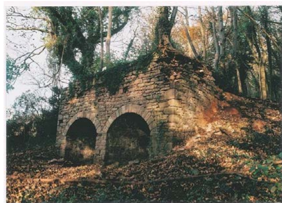
Damage to lime kiln due to vegetation growth – root system forcing out stonework – long standing issue but damage is active and ongoing
