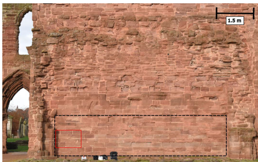
Figure 3. Image of the studied façade at Arbroath Abbey. Black box outlines the boundaries of the area analysed by the moisture meter, and the red box outlines the boundaries of the area that previously had a hydrophobic treatment.
