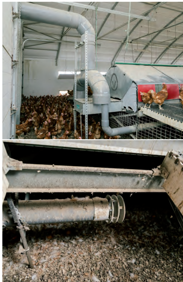
Image 9: Illustration of an ammonia scrubbing system in a poultry house, showing ducting, and air inlet immediately above the manure (Housing Measure 17). In the system shown, ammonia is recovered for use as a fertilizer (see Nutrient Recovery Measure 5) (photographs: © UVA, 2020; ammoniatrapping.com).
