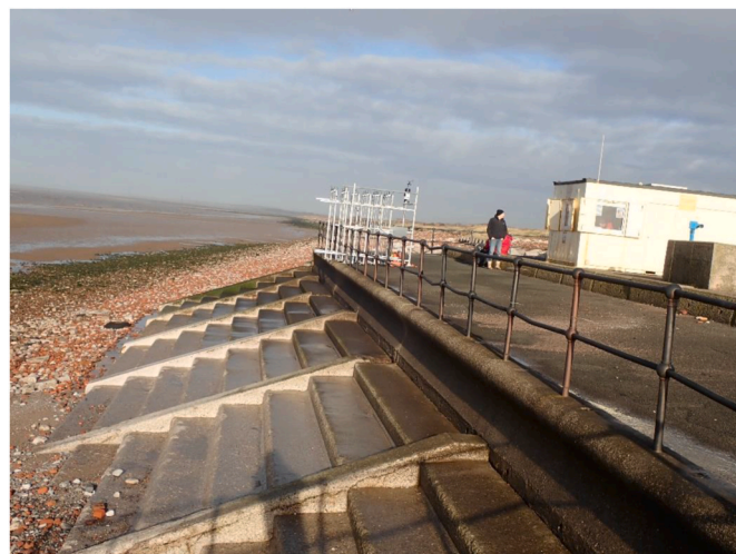
Fig. 2. Photo of the coastal defence at Crosby with foreshore exposed at low tide.
