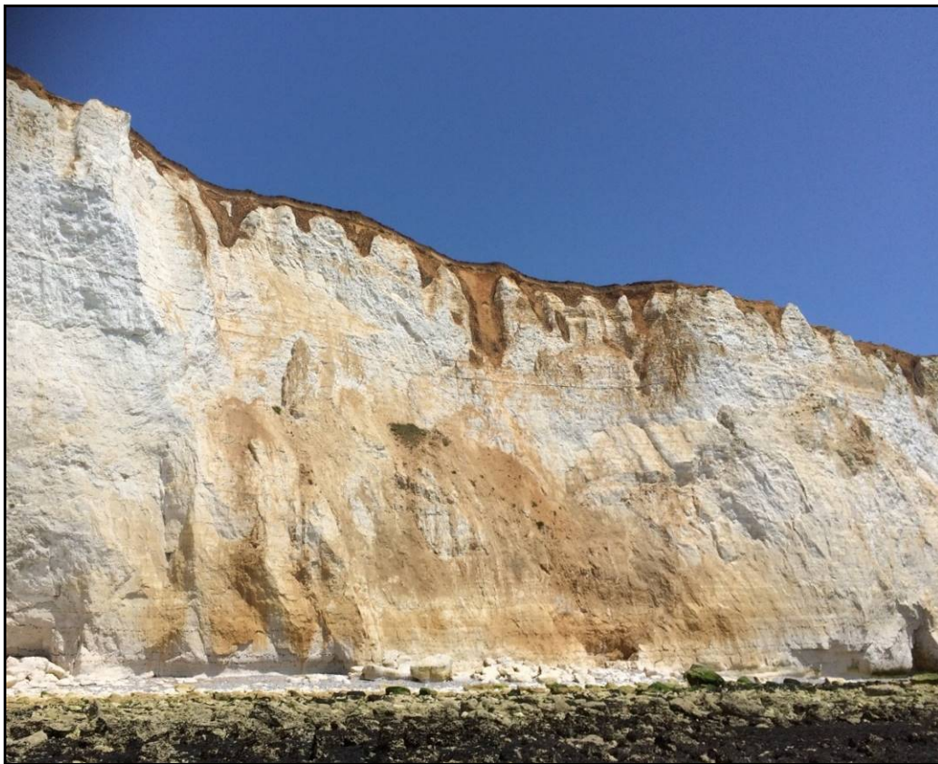
Figure 6. Dissolution pipes infilled with reddish brown sediments developed beneath the Clay-with-Flints, forming an irregular rock-head at the top of the cliff, Seaford Head. Cliff height ~70 m.
