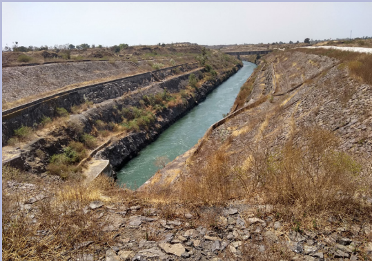
Canal Offtake from Indira Sagar Dam, Madhya Pradesh (Photo credit: Nathan Rickards)
