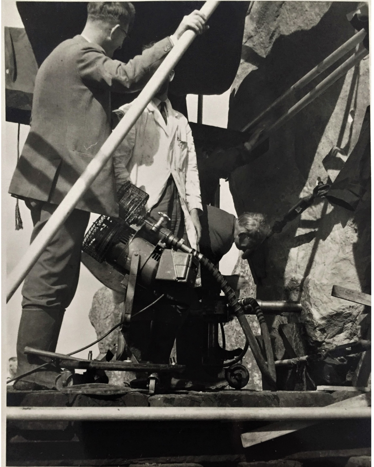
Fig 2. Drilling work on Stone 58 at Stonehenge by Van Moppes Ltd in August 1958, with Mr Robert Phillips pictured left. Permission was obtained from Mr Lewis Phillips for the image of his late father to appear in this picture and for him to be identified by name. This image is reproduced under a CC BY 4.0 license, with permission from Lewis Phillips, original copyright (2020).
