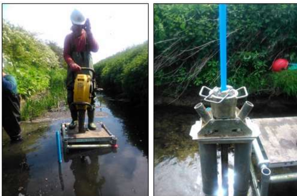
Figure 17 Using the jackhammer for installation. A small podium was used in the river to ensure safe footing while handling (left). Lever-system (levers on not attached yet) to extract the outer metal pipe (right).
