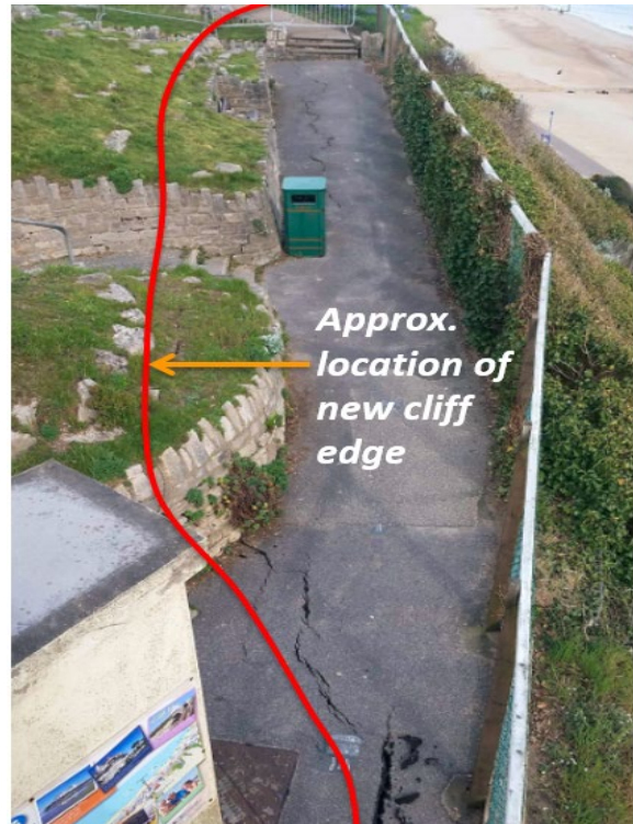
Figure 2 View of the public pathway leading to the beach front on top of the East Cliff, where the landslide incident took place in 2016. Red line denotes the new edge of the cliff after the incident.
