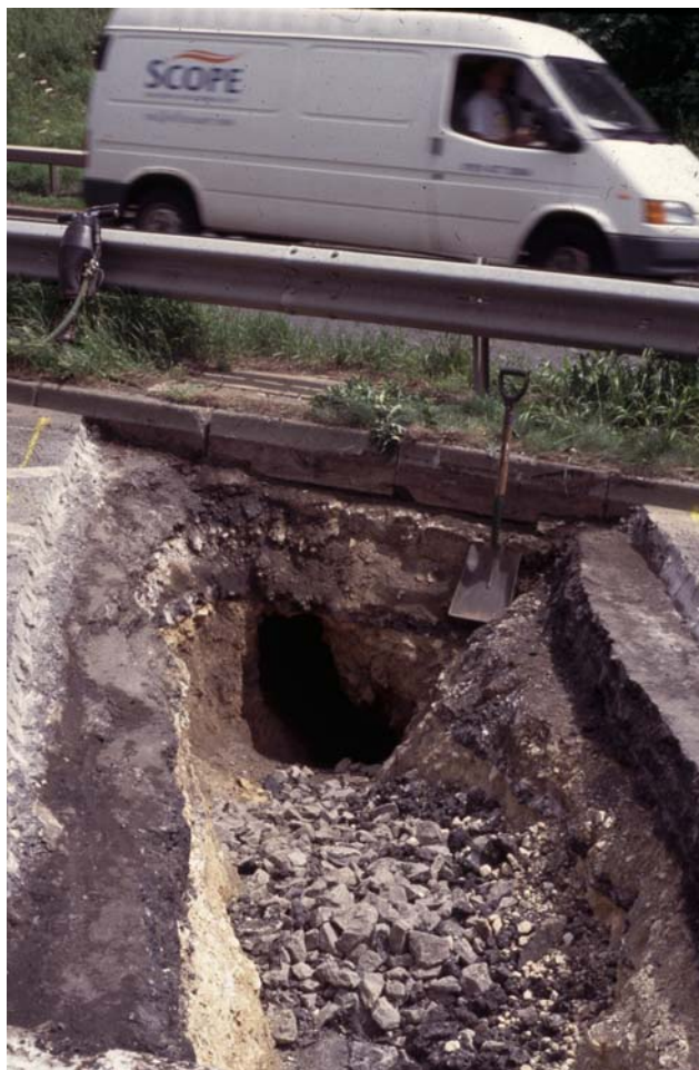
Figure 5. Open fissure immediately beneath tarmac, exposed in excavation of the outside lane of the north-bound carriageway of A 690 road, during repair work 23 June 2003.
