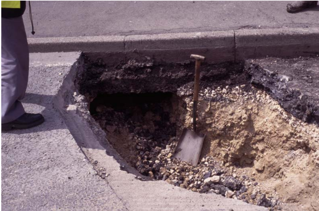
Figure 1. Void beneath pavement, adjoining north-bound carriageway of A 690 road, exposed during repair work 20 June 2003.
