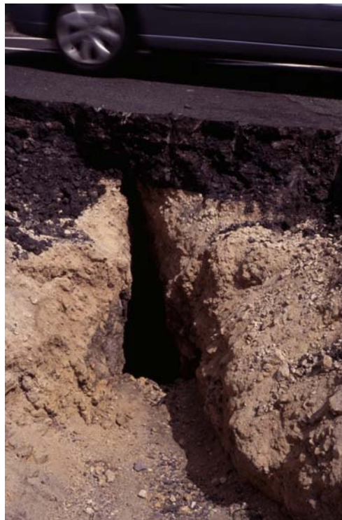
Figure 4. Detailed view of the open fissure immediately beneath the tarmac, seen in Figure 3.
