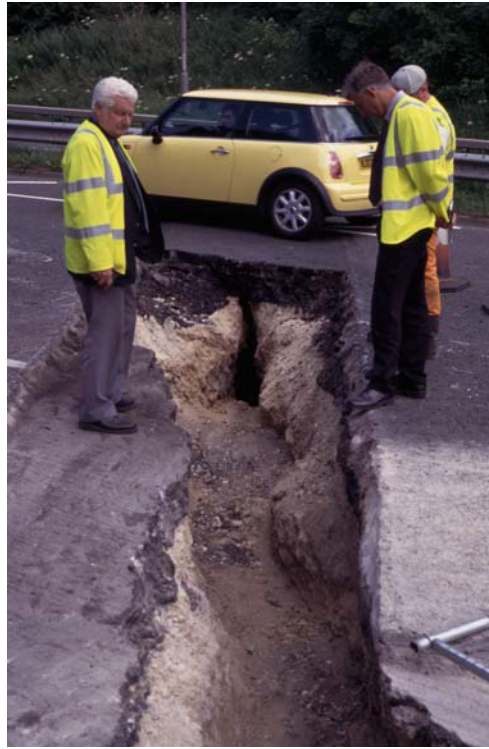
Figure 3. Fissure exposed beneath near-side lanes of north-bound carriageway of A690, 20 June 2003. Walls of solid dolomitic limestone and open fissure beneath tarmac can be clearly seen.
