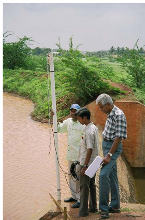
Installation of automatic water level recorder
