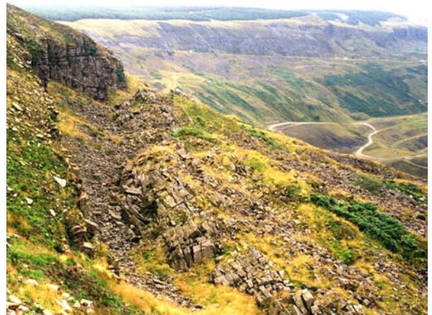
Figure 3 Vertical cliffs in well jointed rock with weaker strata below may fail by pivoting forward, or toppling, as the weaker base crushes. The failure at Garreg Lwyd in the Rhondda Fawr valley is a good example.
