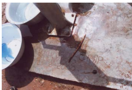
Plate 3. Details of World Vision (WV) Bh 1502 on well head plinth
