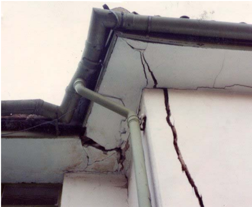
Figure 4 – Structural damage to house caused by ‘end lift’ (© Peter Kelsey & Partners)
