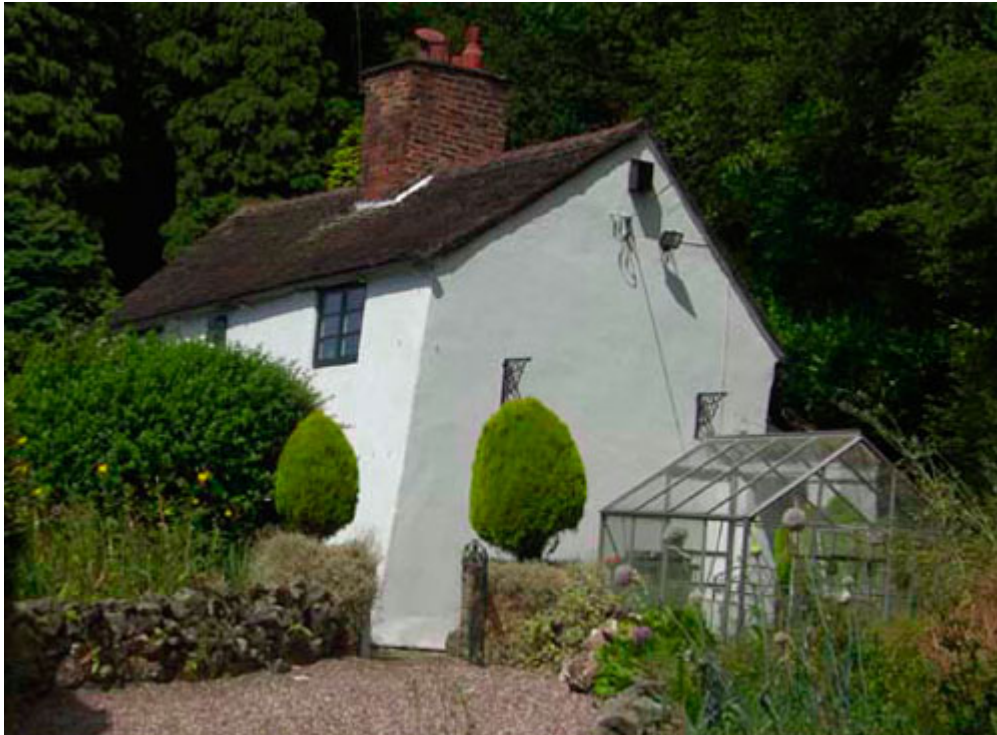
Figure 7 Movement of a house within the Lloyd's Coppice landslide. The greenhouse is vertical.
