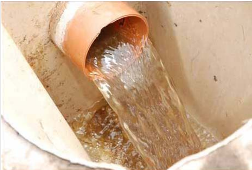
Plate 1 Effluent from a septic tank discharging into an inspection tank
