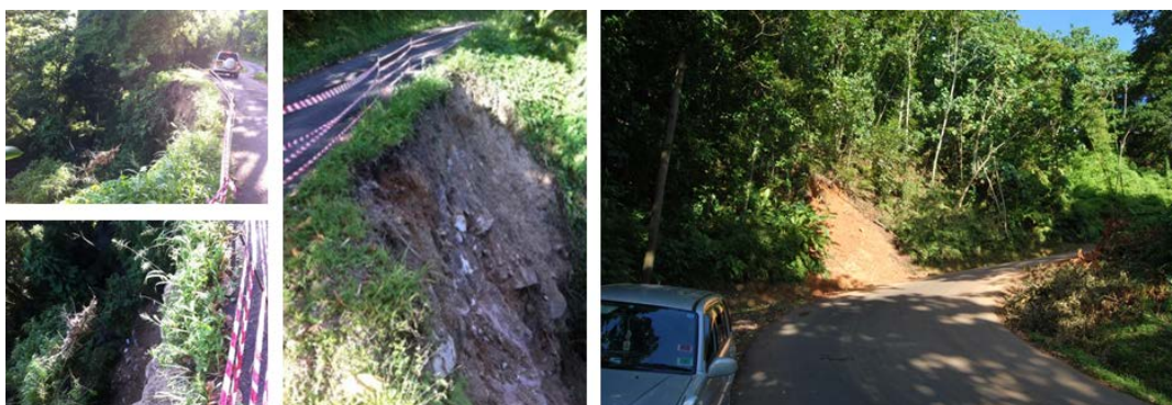
Figure 33. Shallow translational and rotational landslides generated by undercutting along the road to Concorde Falls and, right, a small roadside failure NE of Constantine. These small failures were generated in 2014 but are not visible on the latest satellite image available for this study as these would have occurred since the images were taken. However, given the dimensions of these events, it is highly improbable that these will be picked up by an EO survey.
