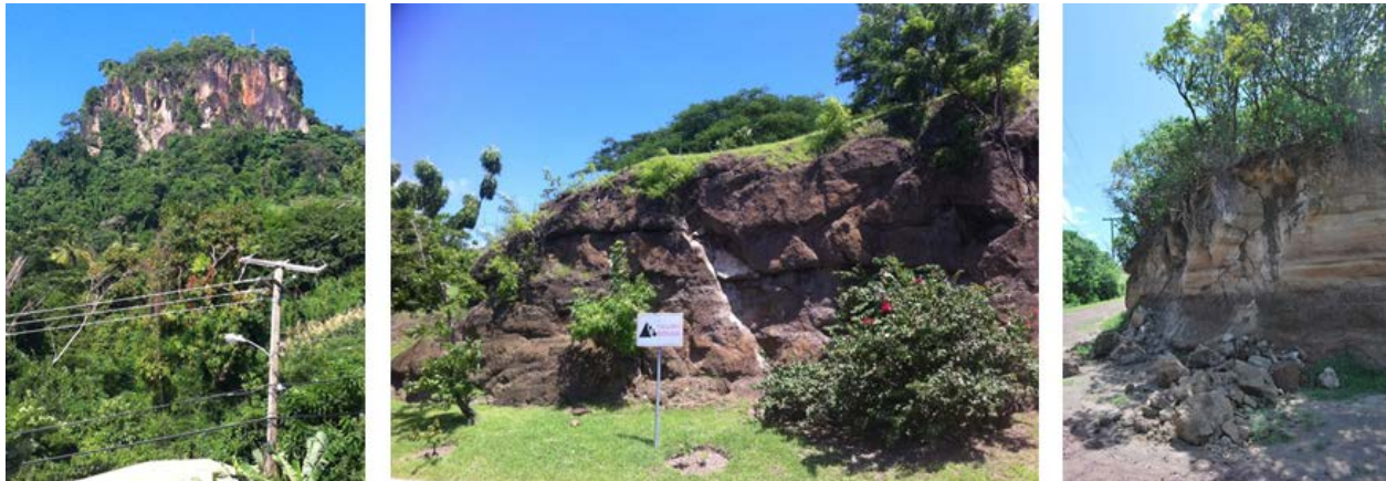
Figure 36. The potential for rockfall is apparent at many sites across the island. A large cliff face near Molinere Point provides an example of many steep cliff faces found throughout the Island from where it is not inconceivable that the occasional rock fall can be generated. Differences in coloration of the cliff faces provide an indication of the dynamic nature of these cliffs. However, dense vegetation along the base of these cliffs will reduce the magnitude of the zone away from the cliff where the effects of rockfalls will be felt. In the absence of vegetation, e.g. near the airport (centre) and along roads (e.g. at Levera, right) rockfalls can pose a hazard with a more direct impact pathway.
