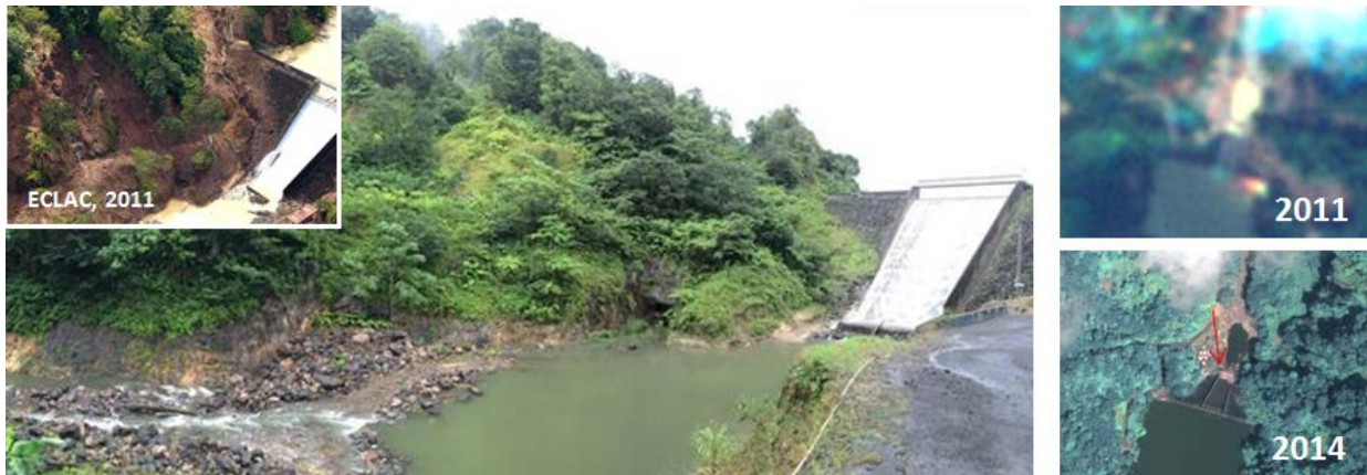
Figure 13 . Landslides near the Roseau Dam. Multiple events in 2010 seriously affected the water quality of the reservoir and a large landslide occurred to the east of the dam (see inset photo from ECLAC 2011). The remains of this landslide are still clearly visible. The direction of the photo is indicated by a red arrow on the satellite image of 2014. Compared with the 2011 image it is evident how much more detail can be observed. Includes material © CNES 2014, Distribution Airbus DS / SPOT Image S.A. France, all rights reserved and material © 2014 BlackBridge, all rights reserved.
