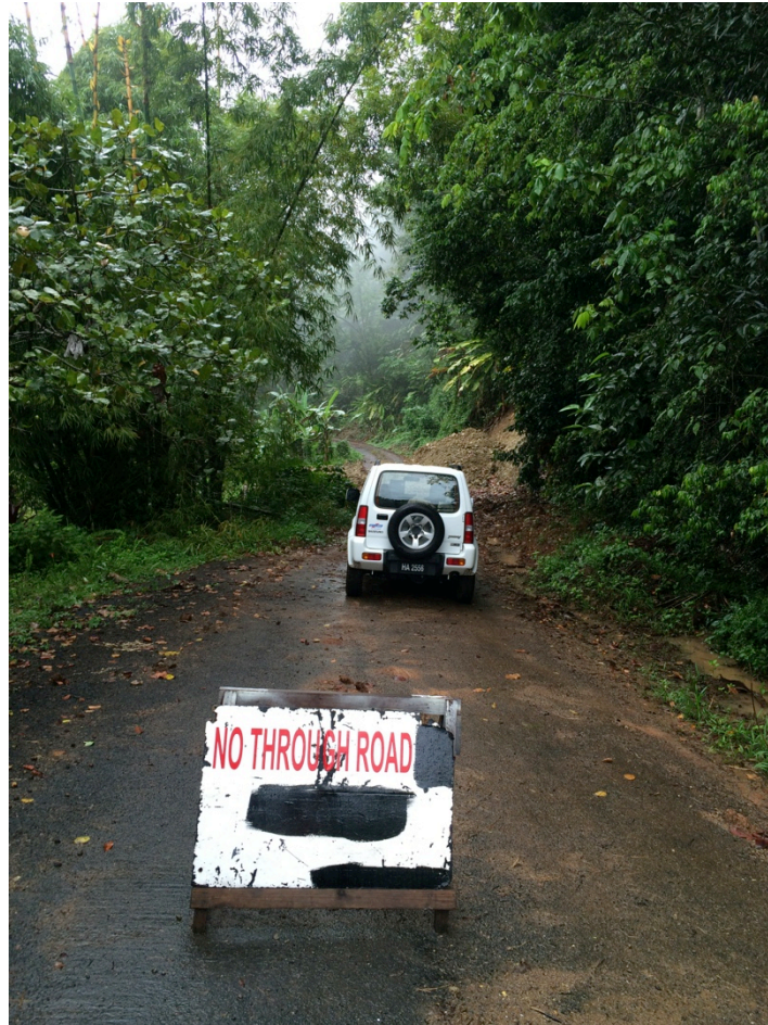
Figure 2 Road closure due to landslides – the type of problem the project is addressing
