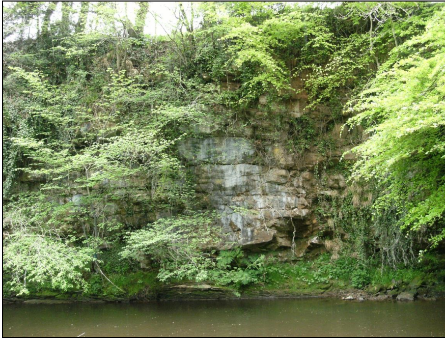
Photo ELC_17 P1: Cliff section on the west bank of the River Esk. The buff coloured sandstone can be seen resting on the softer mudstone/siltstone which is undercuts the sandstone. © BGS, NERC.
