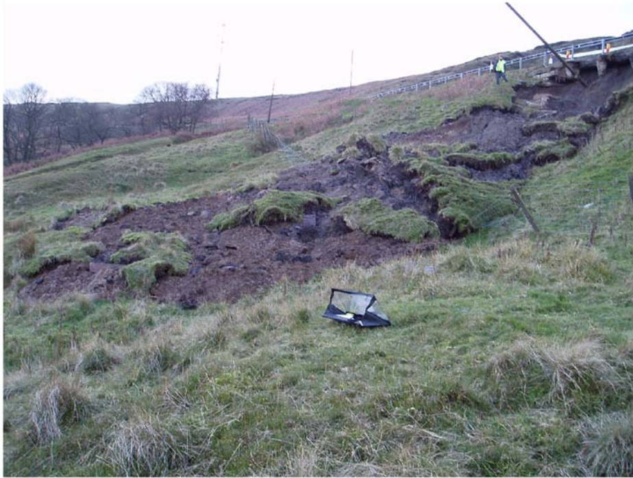
Figure 3-2. Close-up view of Little Hey landslide detail. Photograph taken from [BNG 4 09851 4 04402], facing 260° (SW) (H.J. Reeves, BGS © NERC 2004).
