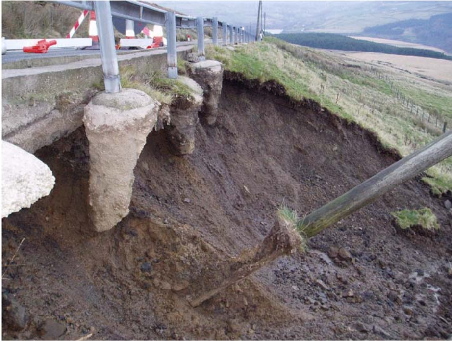
Figure 3-4. Undercutting of the A6024 due to the slope failure at Little Hey landslide. Photograph taken from [BNG 409861 404401], facing 030° (NE) (H.J. Reeves, BGS © NERC 2004).
