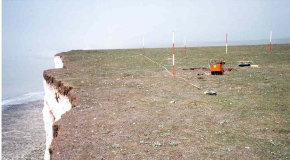
Figure 20. View of Birling Gap Site A in May 2002. The surveyor’s tape hanging over the cliff edge indicates the extent of the cliff lost in the fall.
