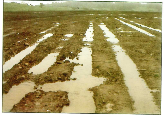
Plate 7 Compaction of topsoil and subsoil during restoration can lead to severe waterlogging problems on restored opencast sites. Careful soil handling, and the use of subsoiling machinery to alleviate compaction, can largely prevent this problem (Photograph J E Good)
