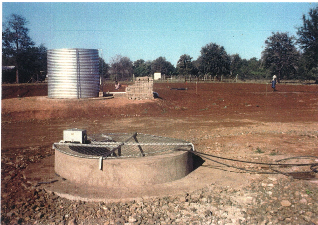
Figure 8. View Showing Well Headworks and Irrigation Header Tank.
