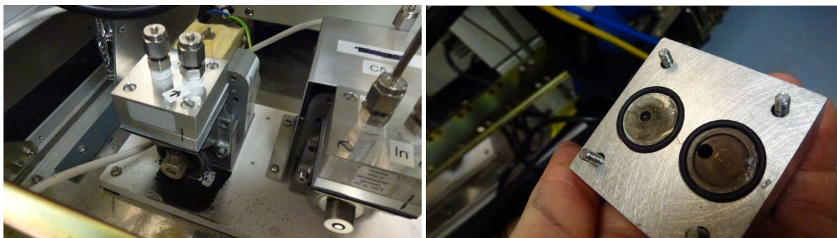
Figure 31: Photographs showing damage to one of the diaphragm pumps as indicated by the black residue (left, below the pump rotating shaft) and the suspected cause of the damage, which was trapped water inside the pump head (right).
