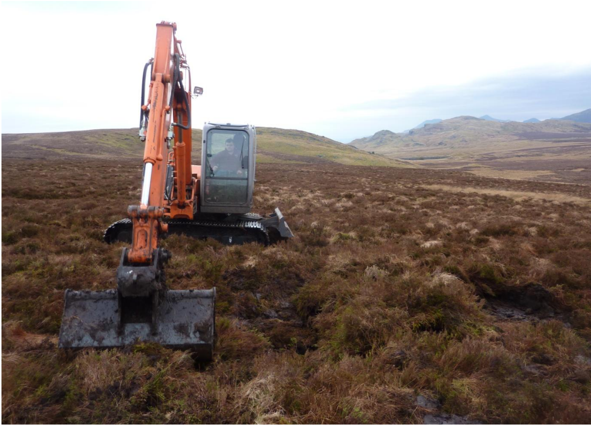
Figure 1. Ditch blocking at the study site in the Afon Ddu catchment.
