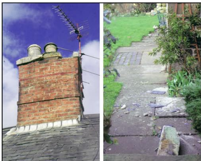
Figure 3. Earthquake damage to John Aram's house, where limestone coping fell from the chimney into the front garden.
