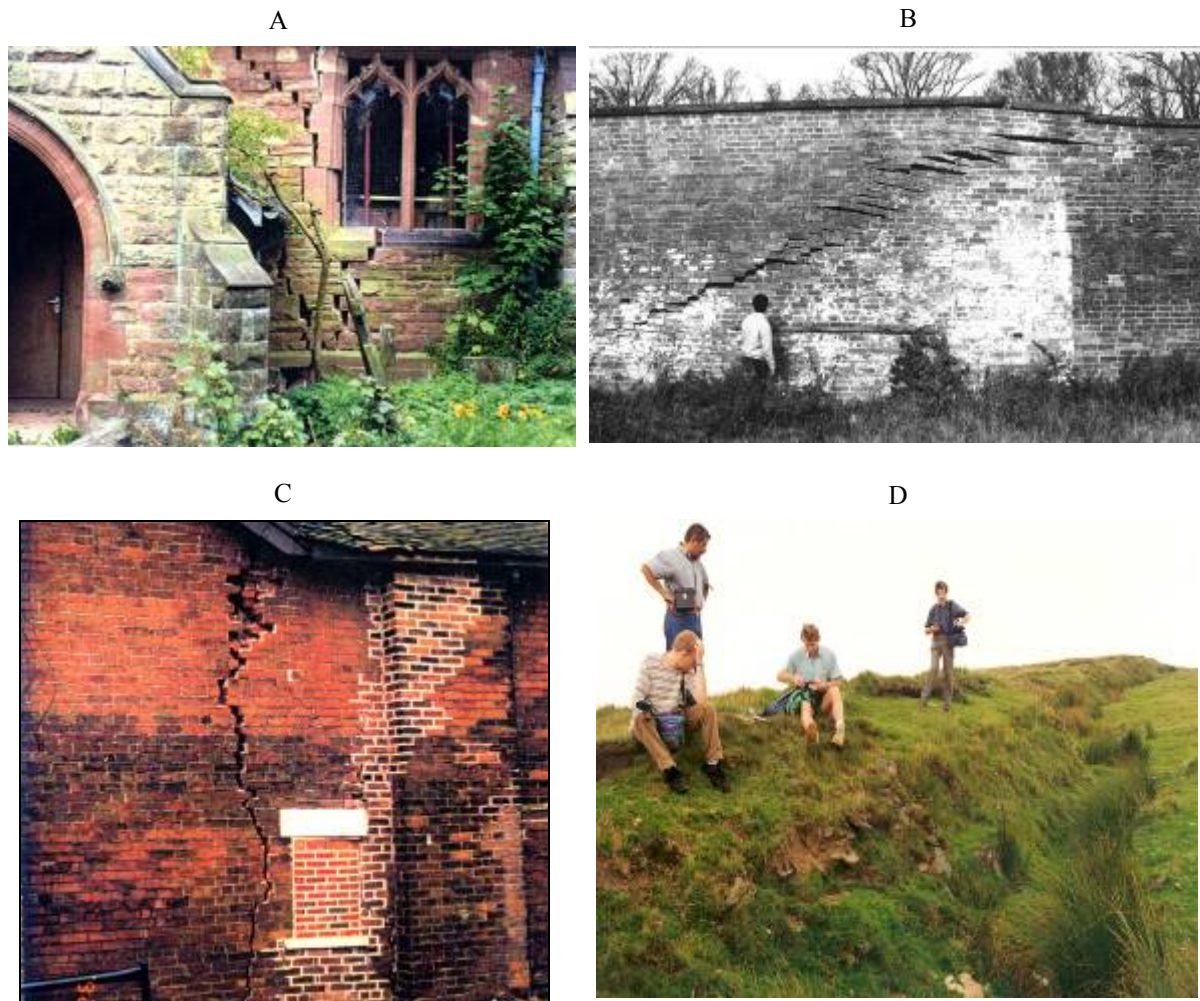
Figure 2 The results of fault reactivation contemporaneous with mining and subsidence. (A) Severe damage to Barlaston Church, Staffordshire. (B) Compression along a fault, Eastwood Hall, Nottinghamshire. (C) A house built on the outcrop of the Hopton Fault, Oulton, Staffordshire. (D) The 4 m high and 4 km long, Tableland Fault scarp wall, at the head of the Ogwr Valley, South Wales. This fault scarp was likely to have originally been generated by deglaciation and stress relief of valley sides in the closing stages of the Pleistocene 'Ice Age' and subsequently exacerbated by mining subsidence over centuries of coal mining (after Donnelly 1994).
