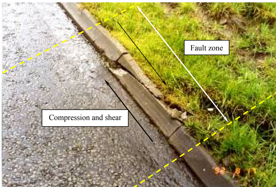
Figure 10. (A) Post mining residual subsidence and fault reactivation ground movements, (B) accompanied by high compressive strains within the fault zones, 10 years after mining ceased, causing damage to the Nelson to Gelligaer road, South Wales (after Donnelly 1994).
