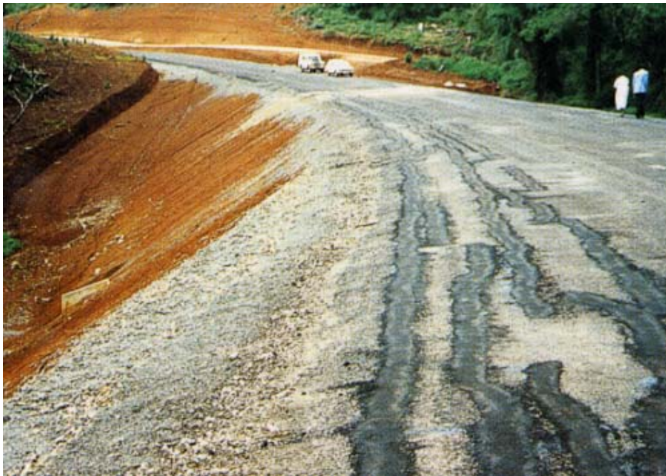
Figure 1. Cracking in a red soil road embankment in Kenya. Cracks up to six centimetres wide have been repaired with asphalt [10]
