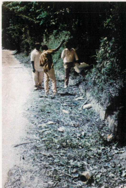
Figure 3.11 Ditch and culvert choked with dirt, leaves and other debris on the upslope side of the main road above Ivy Store landslide. Increased groundwater flow into the slope due to blockage of these water channels and increased run-off from the metallised road surface, may have been critical factors in triggering the landslide downslope of the road. The people in the picture are inspecting a cracked and displaced retaining wall, indicative of further movements in the steep slope above the road.
