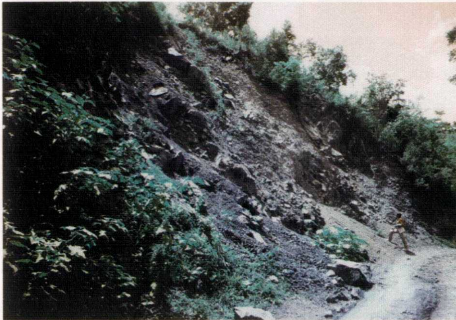
Figure 3.6 Translational debris slide in weathered and fractured rocks of the Arthurs Seat Formation, adjacent to the Crawle River-Arthurs Seat Road. Over-steepening and removal of support from steep sideslopes due to road cutting results in frequent slope failures of this type.
