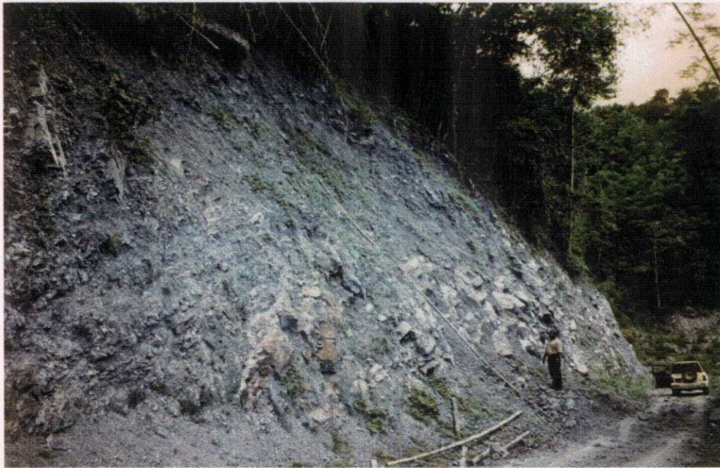
Figure 3.5 Small scale rock and debris fall from a steep road cut in volcanoclastic sediments of the Bullhead Formation, Main Ridge. Debris, recently cleared from road, is derived from the weathered, fractured and jointed bedrock and overlying, 1-2m thick, colluvium comprising earth and rock fragments.
