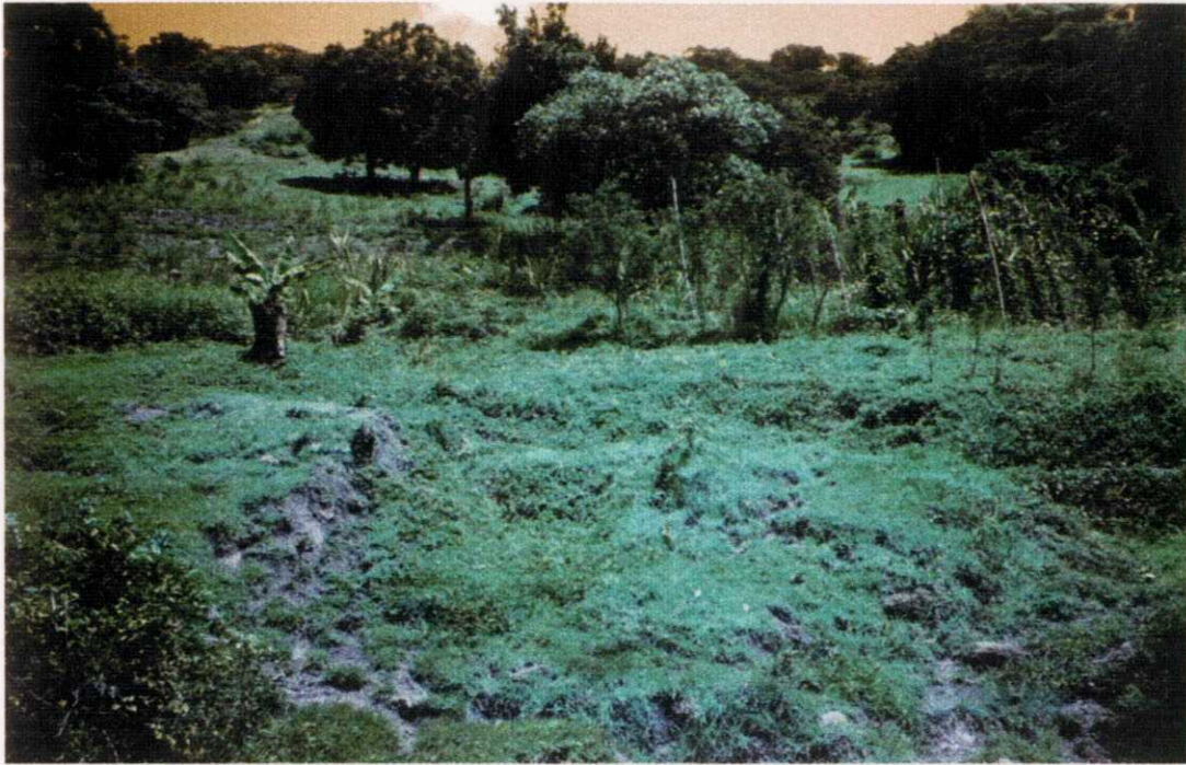
Figure 3.9 Complex earth-slide on a cultivated slope adjacent to the Crawle River-Arthurs Seat road. The slide has occurred in Diamonds Gravelly Clay Loam, overlying weathered shales and volcanic grits of the Arthurs Seat Formation. The entire slope shown in the figure shows evidence of active movement. A small, wet, active earth slide is seen in the toe area in the bottom centre of the figure. To the right, not shown, trees lean severely downslope as a result of recent movements.
