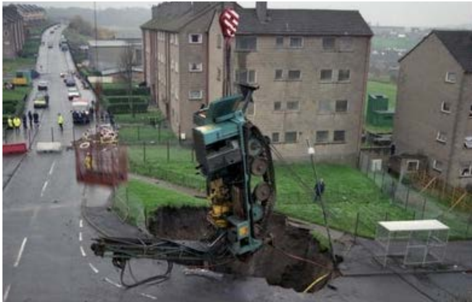
Fig 2 Collapsed mineshaft Garsgadden Mine.
