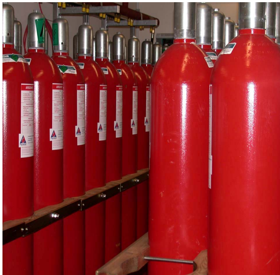
Fire suppression system, NGRC Keyworth
