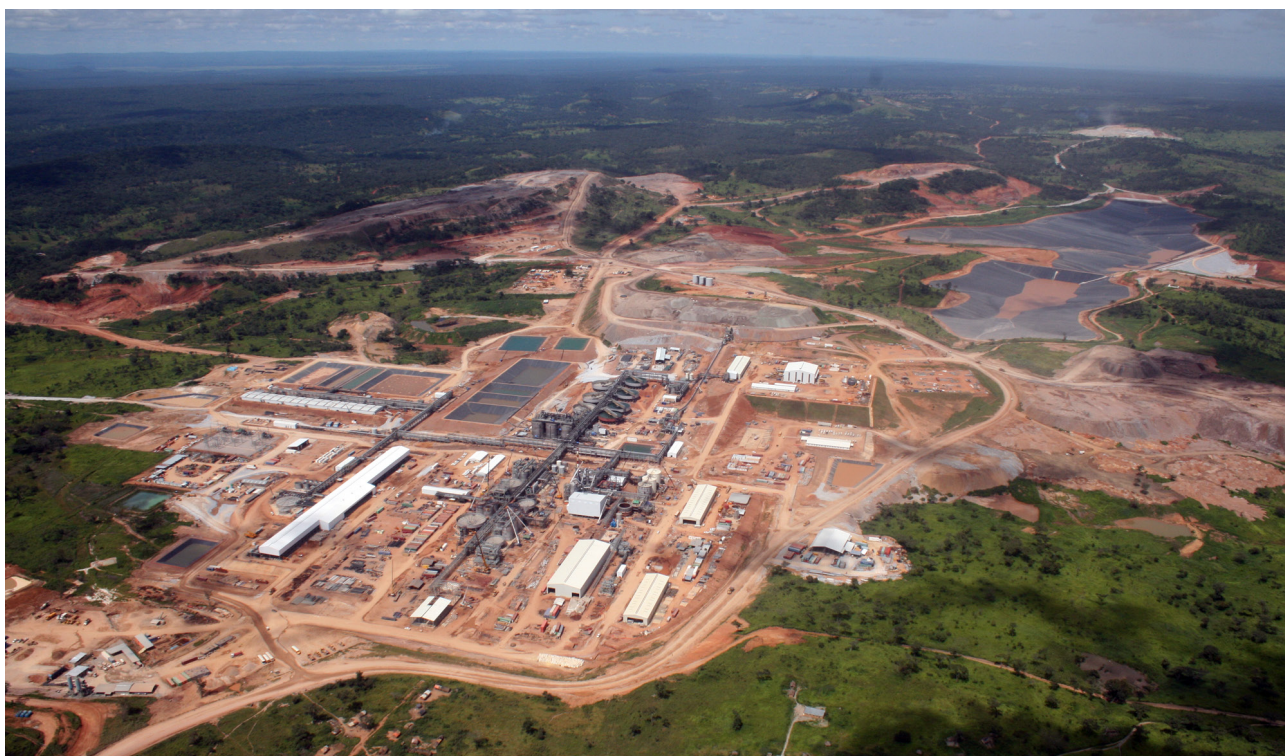
Figure 7 Construction of the Tenke Fungurume operation, a copper-cobalt deposit located in the Democratic Republic of Congo. Courtesy of Freeport McMoRan Copper and Gold Inc.
