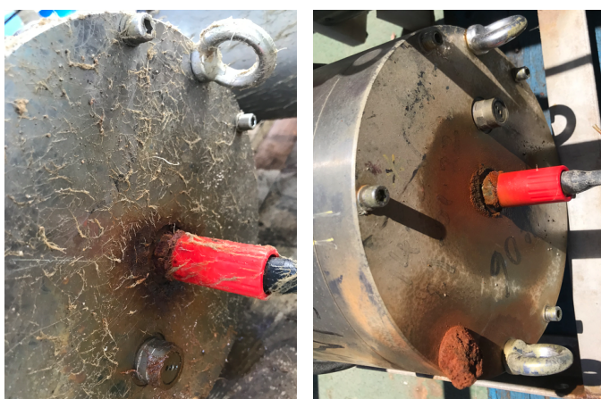
Figure 12.5 Evidence of bulkhead corrosion on titanium battery housings.
