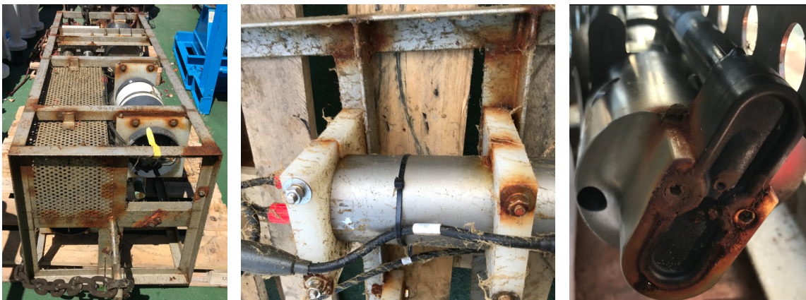
Figure 12.3 Examples of corrosion on the frames and instruments.
