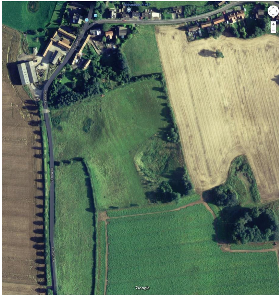
Figure 47. Aerial Photograph of surface depressions around [SE 32421 73149] as shown in Cooper (1989) affecting an area of glacial till over Sherwood Sandstone Group near Hutton Conyers ( https://goo.gl/maps/fY4ZDjM4kny )
