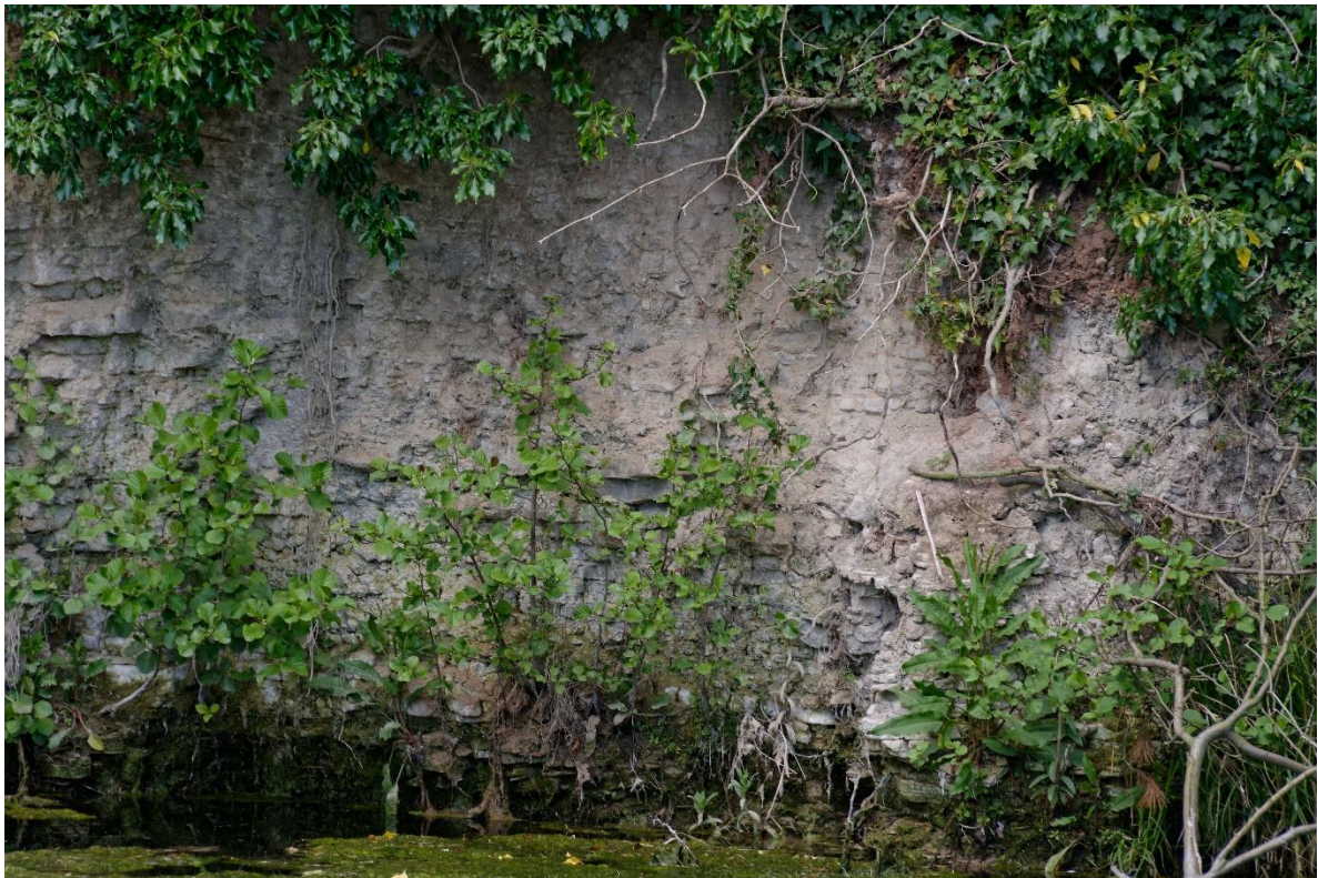
Figure 69. Brotherton Formation limestone in the back wall of the 1939 Hall Garth Ponds doline (sinkhole).
